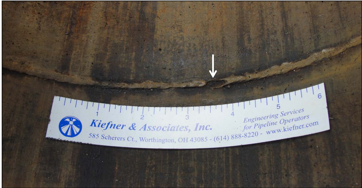
Figure 16. Burn-through Feature, Weld 026
