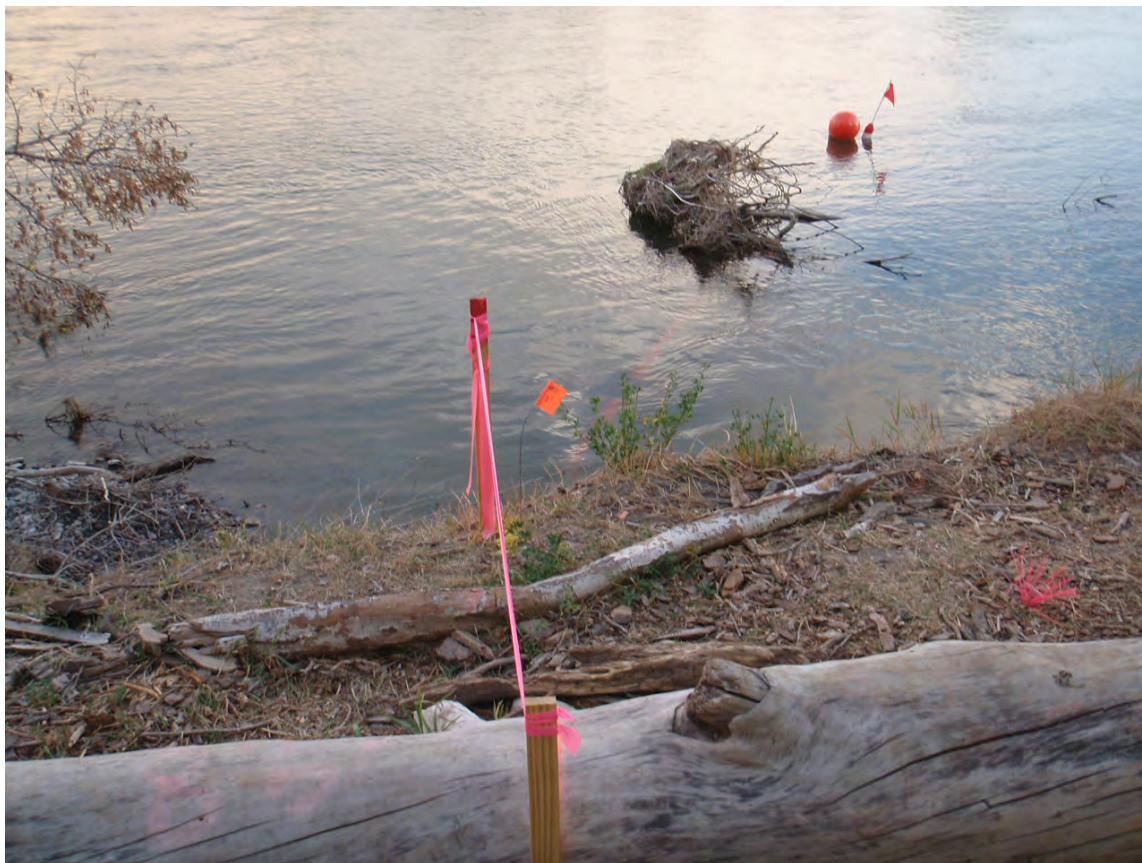
Picture taken from the south bank looking north on Thursday, September 29, 2011, 2:55:09 PM. One can see the pipe deflection downstream under the water. The buoy is marking the north end of the ruptured pipe from the south bank. The two lath tied together with pink ribbon are in line with the original pipeline right-of-way alignment from south to north. One can see a root ball that appears to be hung up on the pipeline. The red abrasive resistant fusion bonded epoxy (FBE) coating can be seen on the pipe. The pipe was originally concrete coated over the FBE coating.
