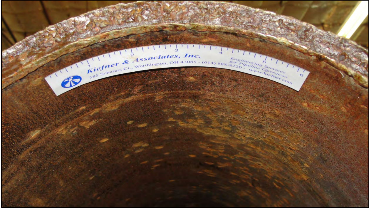
Figure 11. Interior Surface Pitting
