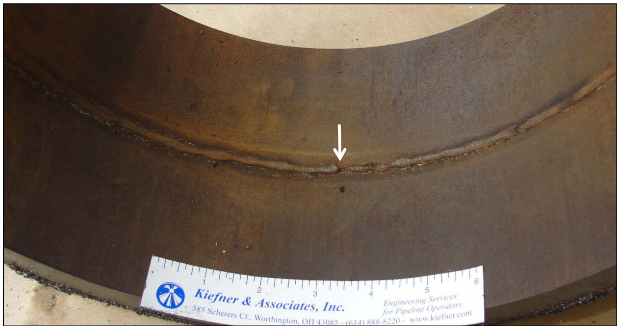
Figure 17. Inadequate Penetration Feature, Weld 030
