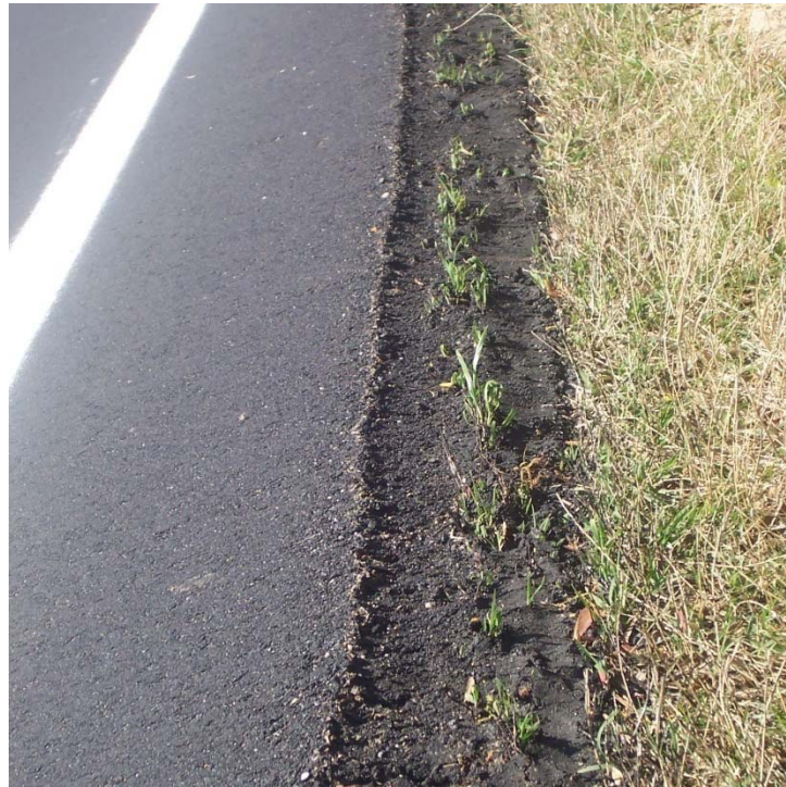
Figure 6. Example of Safety Edge SM placed on heavy vegetation – due to lack of adequate compaction the Safety Edge SM will deteriorate.
