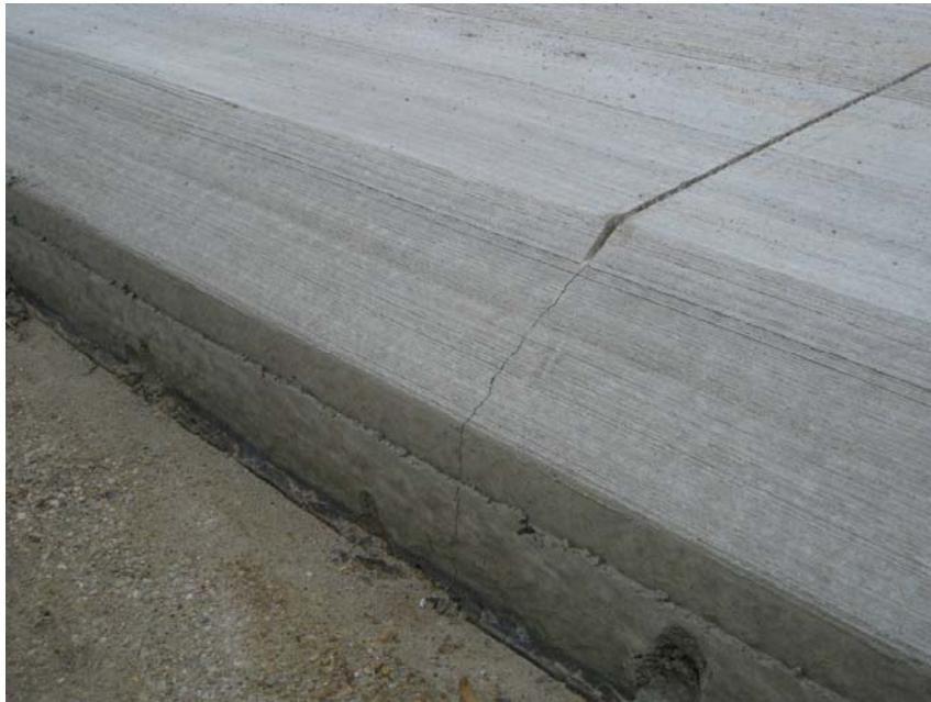
Figure 16. Sawcut and crack at the formed joint on one of the Safety Edge SM demonstration projects.
