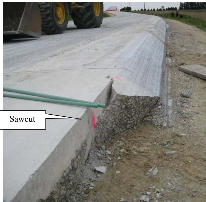
Figure 4. Sawcut on a PCC project at an intersection to remove the Safety Edge SM .
