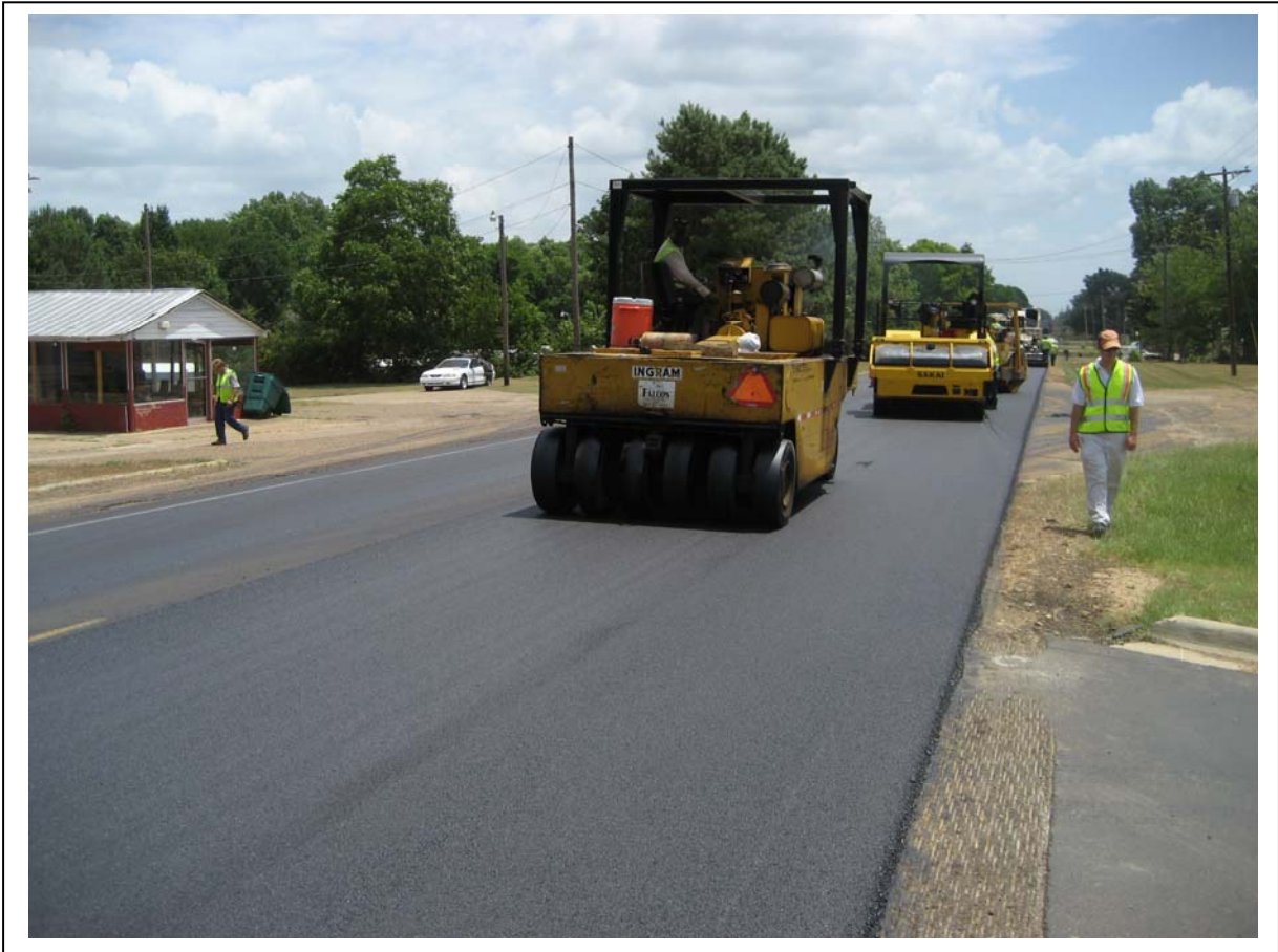
Figure 13. Rolling the Safety Edges SM with standard rollers – No special rollers are required.
