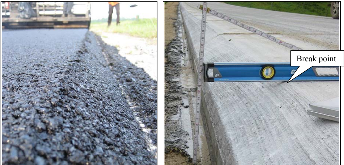
(a) AC Project.
