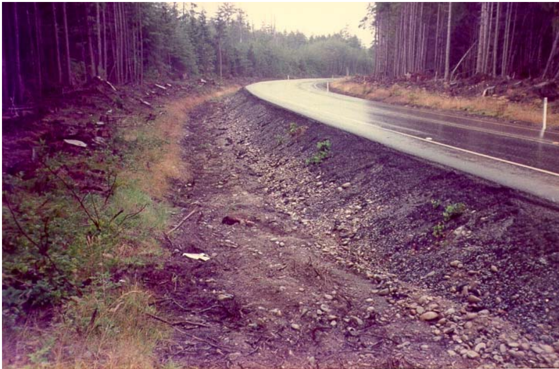
Figure 2. Example of where a foreslope/embankment is too steep for the Safety Edge SM .
