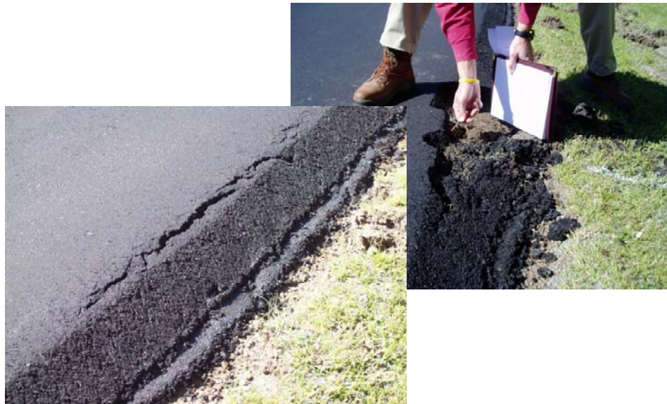
Figure 11. Longitudinal crack due to Safety Edge SM break point located on unimproved shoulder.
