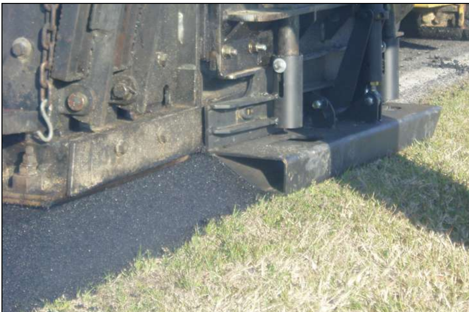
Figure 12. Safety Edges SM directly behind the Carlson device.
