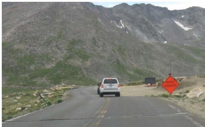
Figure 4-27. Mount Evans Highway road damage, summer 2012.
