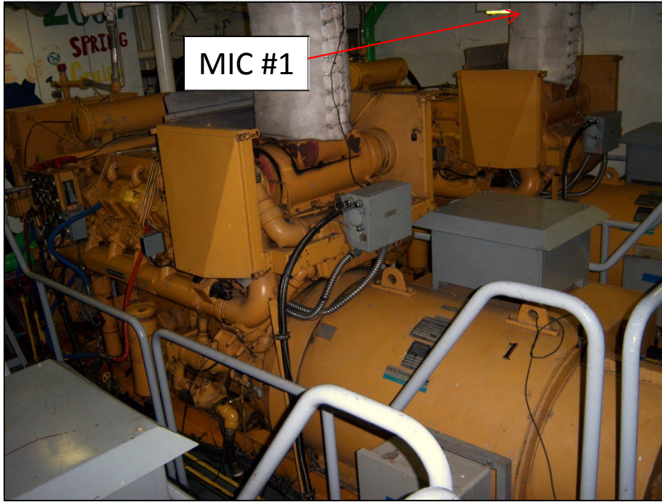
Engine Room Layout – Diesels #1 and #3 Looking Forward and Starboard (MIC #1)
