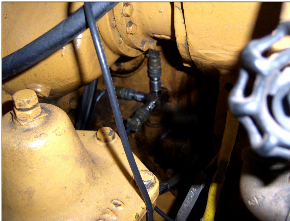
Main Diesel AFT BEARING
