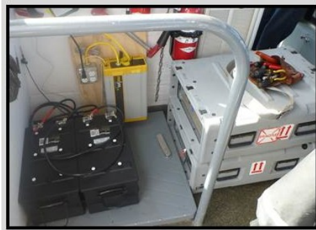
Power and Array Interface Boxes
