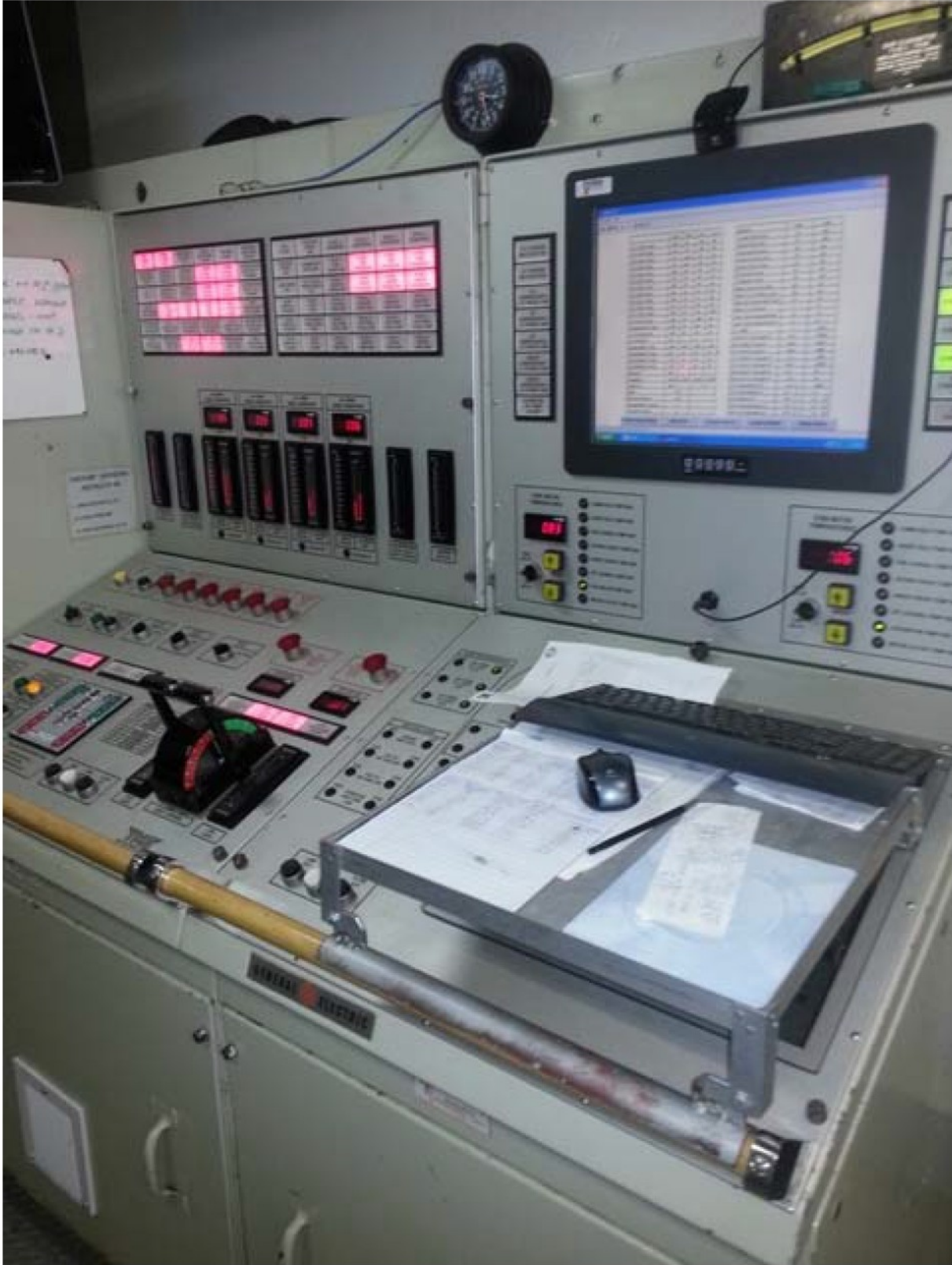
Figure 7. Engine Room Machinery Control Station
