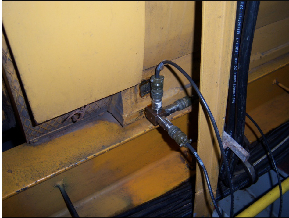
Generator Coupled End Bearing
