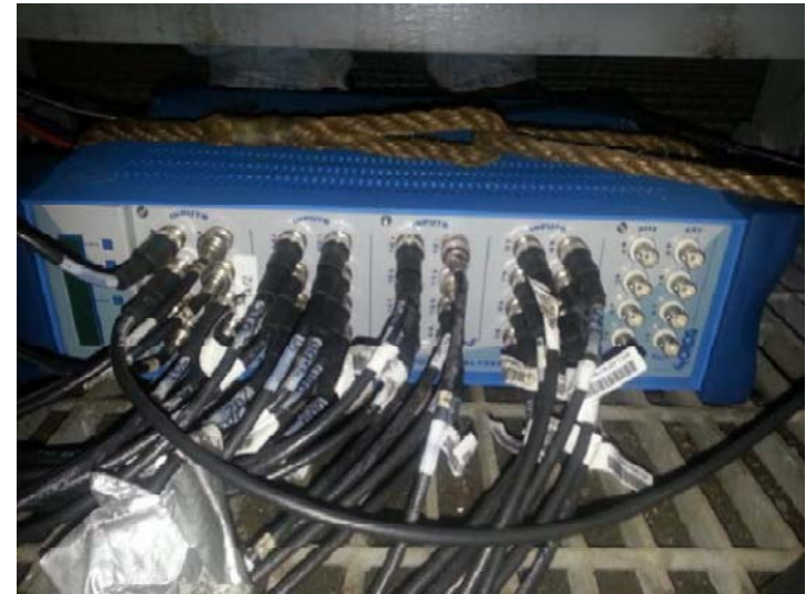
Data Recorder – Engine Room
