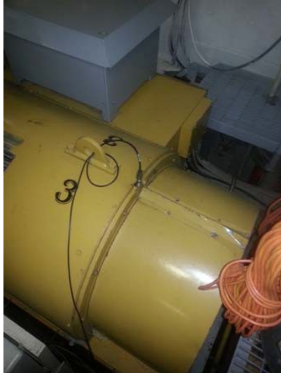
Figure 16. Generator Aft Accelerometer
