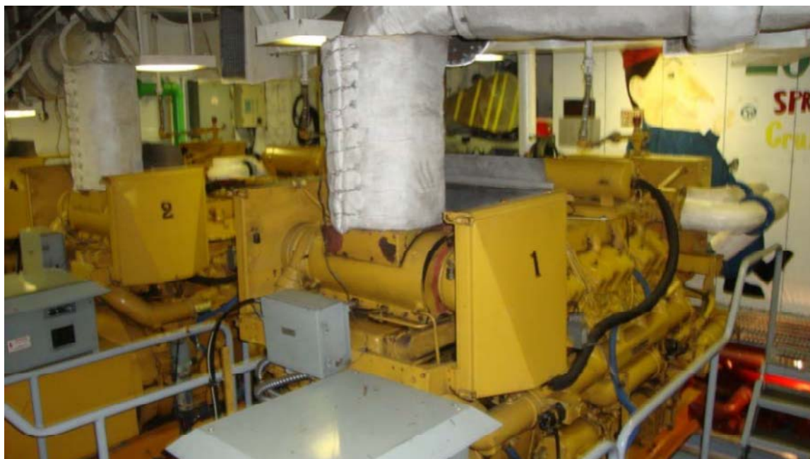
Figure 2-3: T/S State of Michigan Engine Room - D398 Generator Sets
