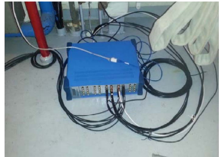
Data Recorder – Motor Room
