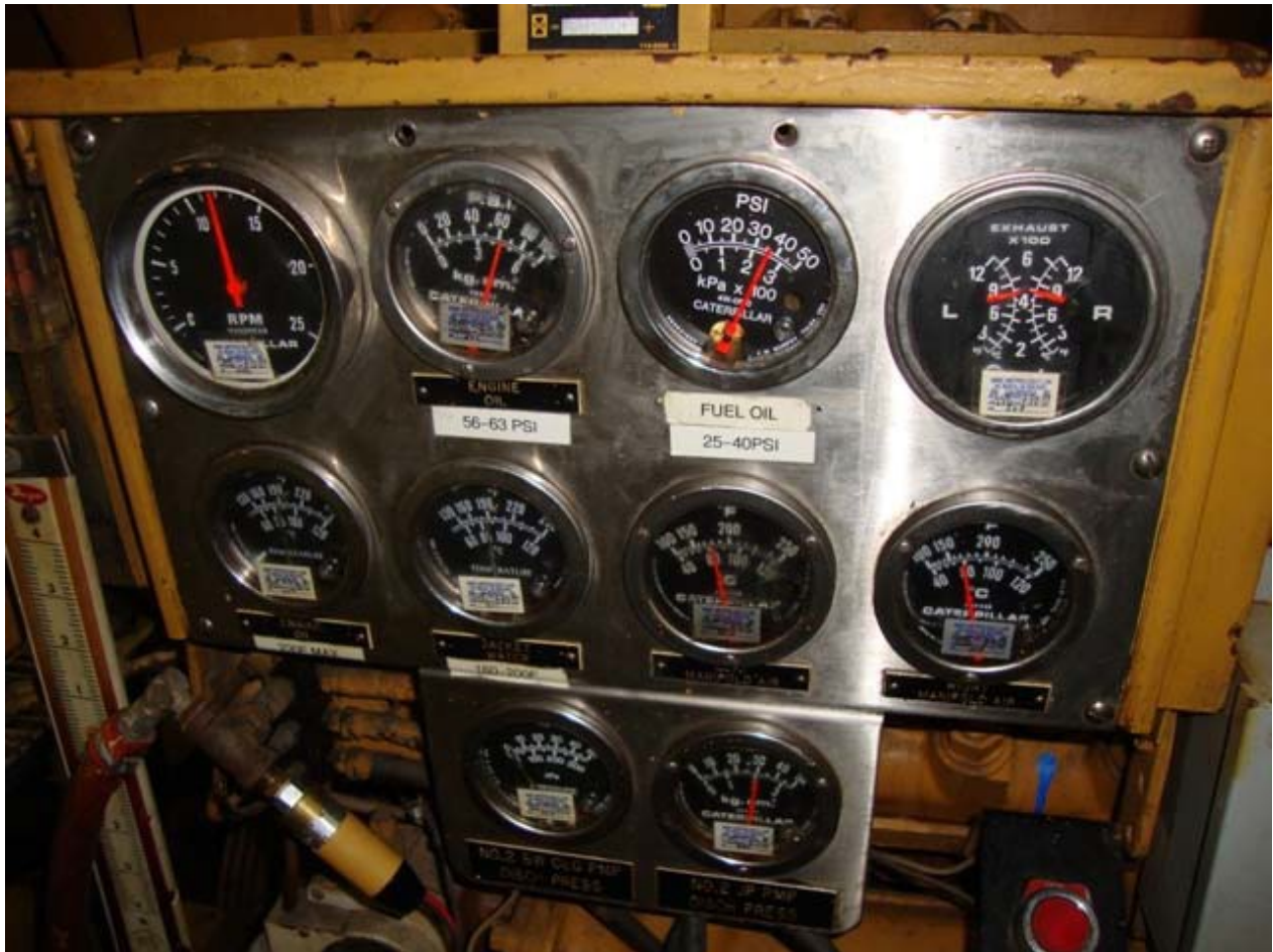
Figure 6. Engine Local Operating Panel
