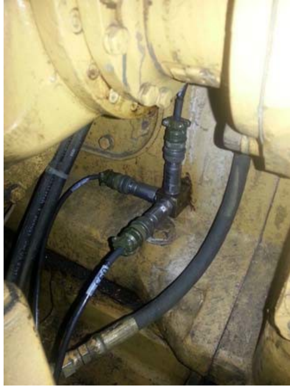
Figure 14. Diesel Engine Aft Accelerometers
