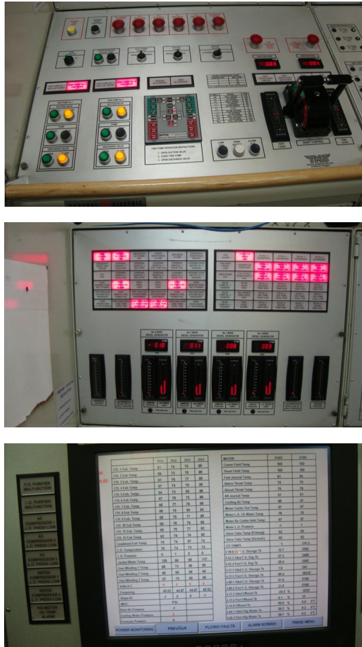
Figure 8. Engine Room Machinery Control Station
