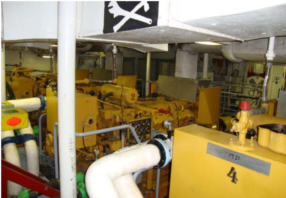
Figure 3. T/S STATE OF MICHIGAN Engine Room
