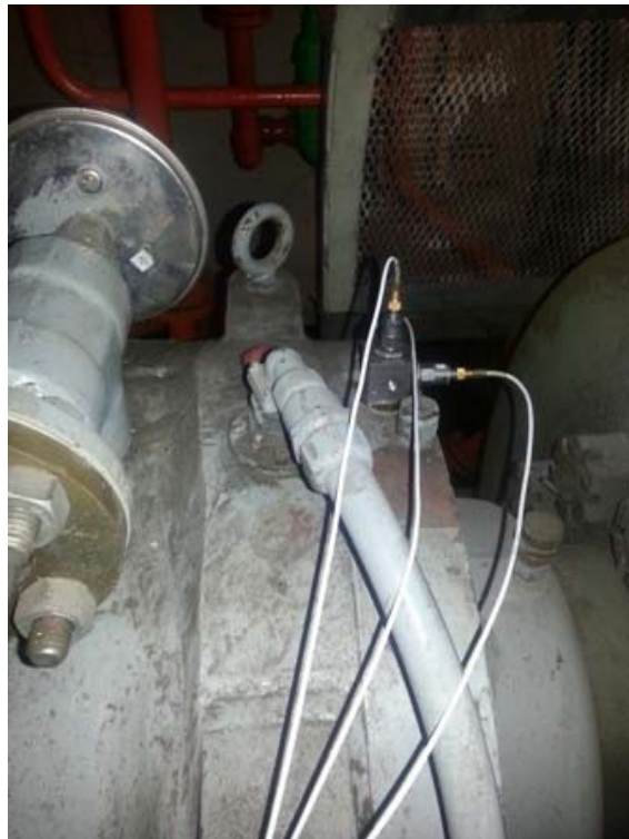
Figure 19. Propulsion Motor Lineshaft Bearing (By Coupling Cover) Accelerometers
