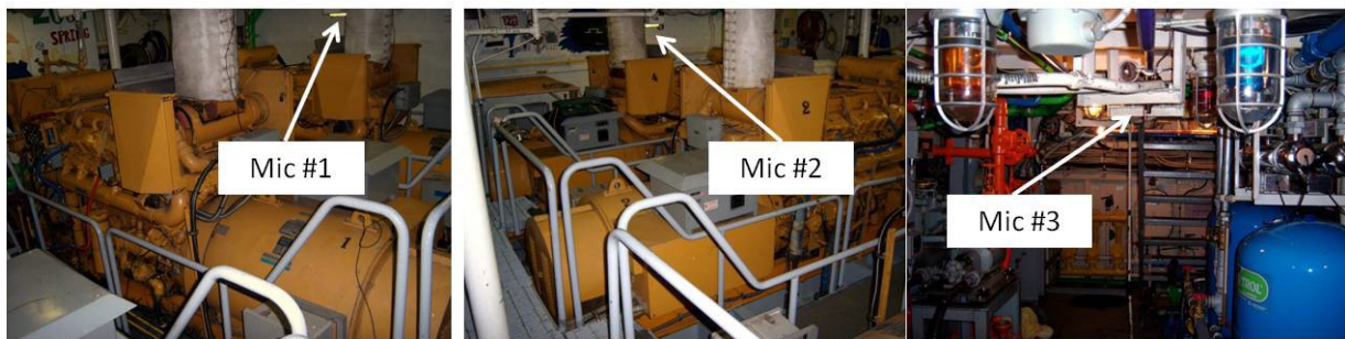
Figure 33. Microphone Installation for Engine Room Sound Measurement
