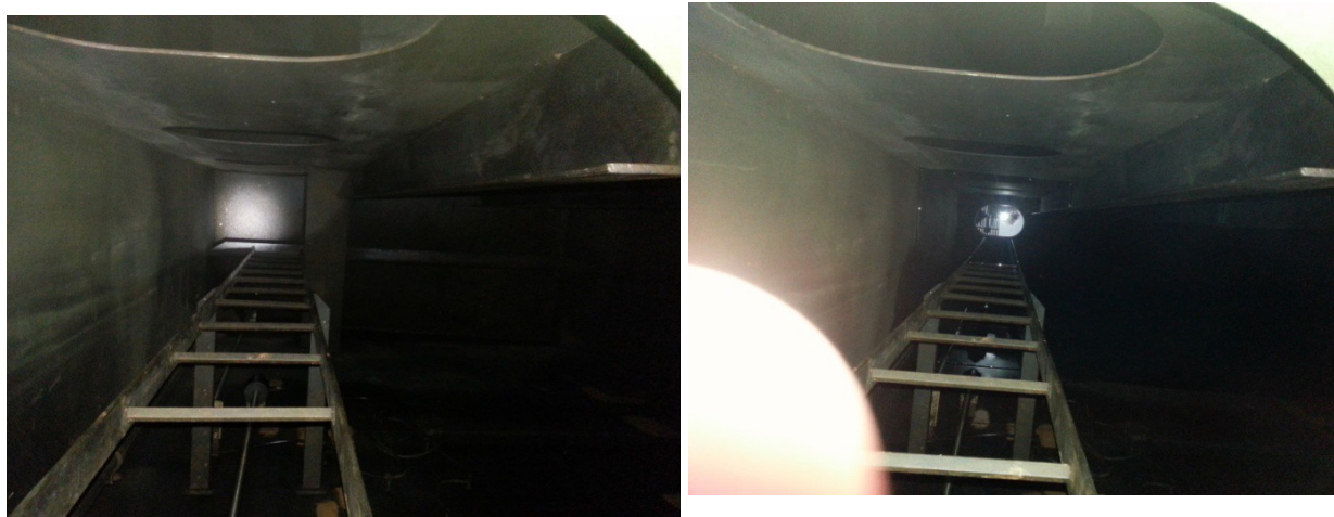
Figure 1. Tank 4-80-2-F-P Tank (empty left – with test fuel added right)
