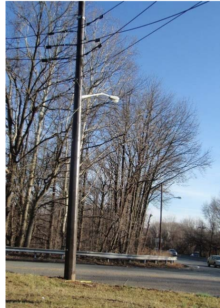
Figure H-2. Photo. NJDOT used utility poles made from fiberglass that would collapse upon impact and not break away into the road.
