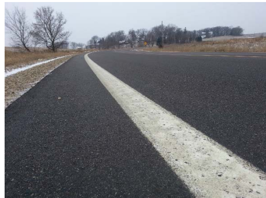
Figure 7. Photo. Delineation with enhanced (6-inch) edge lines.
