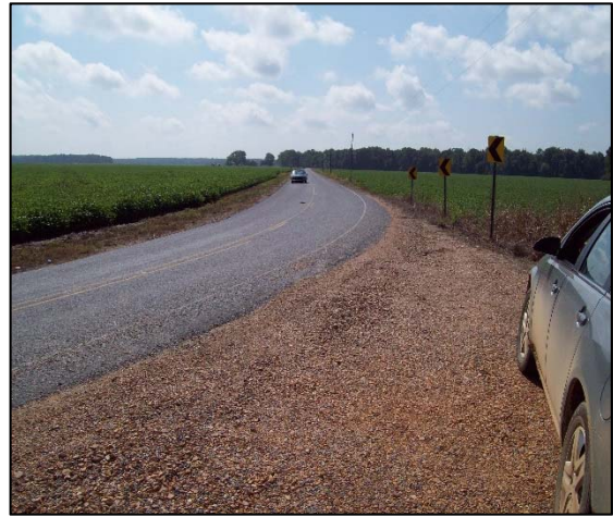
Figure 68. Photo. Intersection with aggregate scattered on paved roadway.
