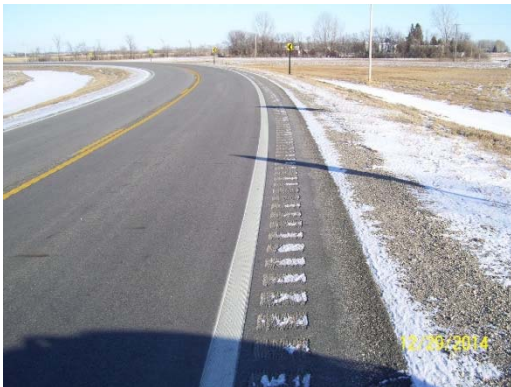
Figure 6. Photo. Adding narrow paved shoulders (2 feet) to existing top width. Includes rumble strips and Safety Edge SM . Source: MnDOT.
