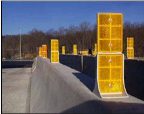
Figure 57. Photo. Delineated concrete barriers. Source: Michigan DOT.
