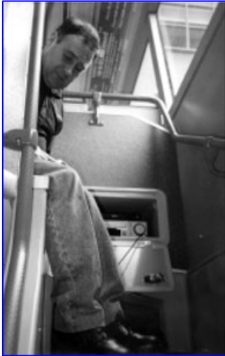
Security cameras can be installed on buses where drivers cannot monitor occurrences.
