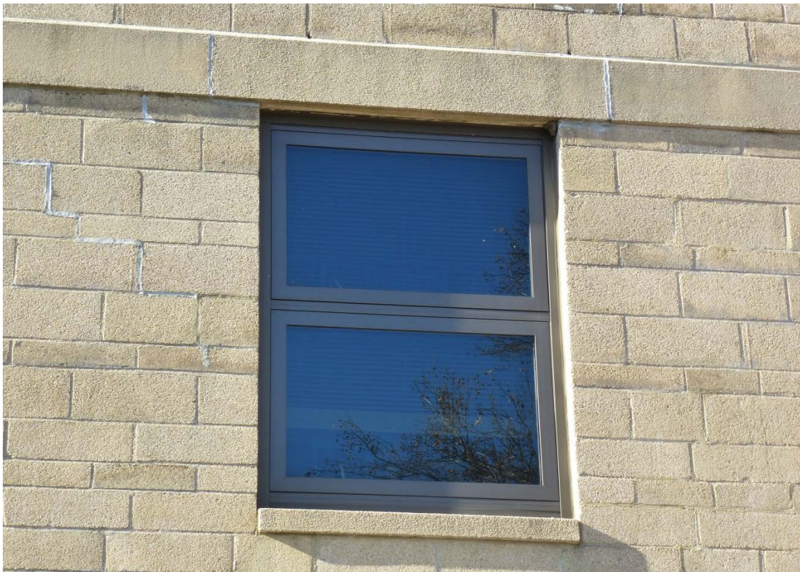
Figure 178. Replacement window with cast-stone belt course above and cast-stone lintel below at Admissions Center (ERDC-CERL, 2013).
