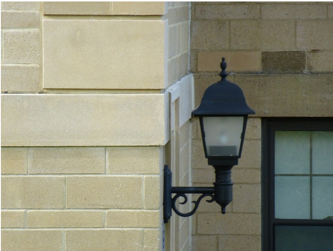
Figure 95. Typical replacement light fixture at entrance to one of the barracks (ERDC-CERL, 2013).
