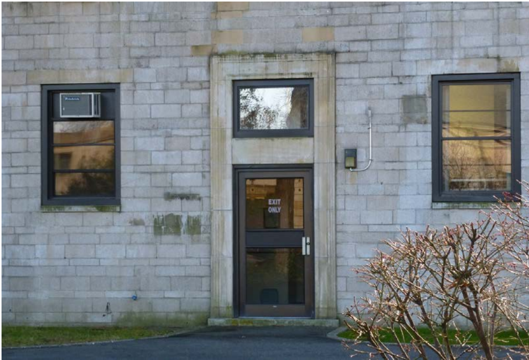
Figure 181. West façade detail of Patten Medical Clinic, showing concrete block pattern and cast-stone surrounds (ERDC-CERL, 2013).
