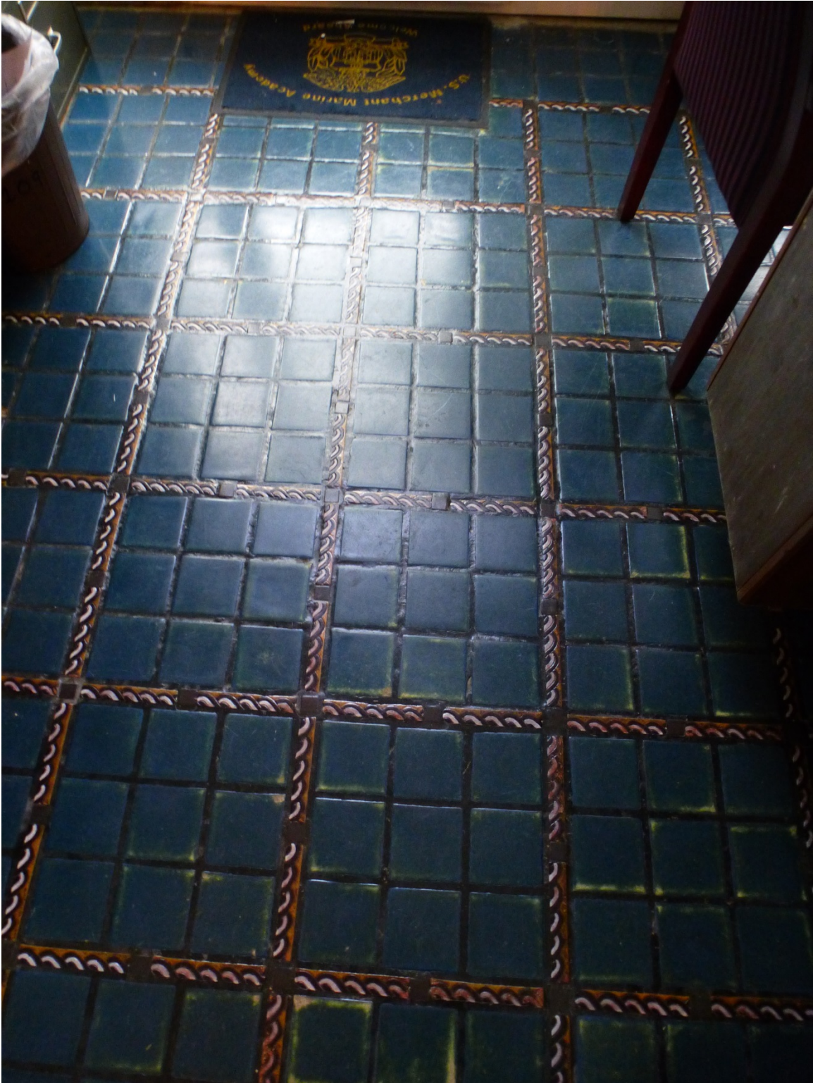
Figure 81. Tile floor in Wiley Hall (ERDC-CERL, 2013).
