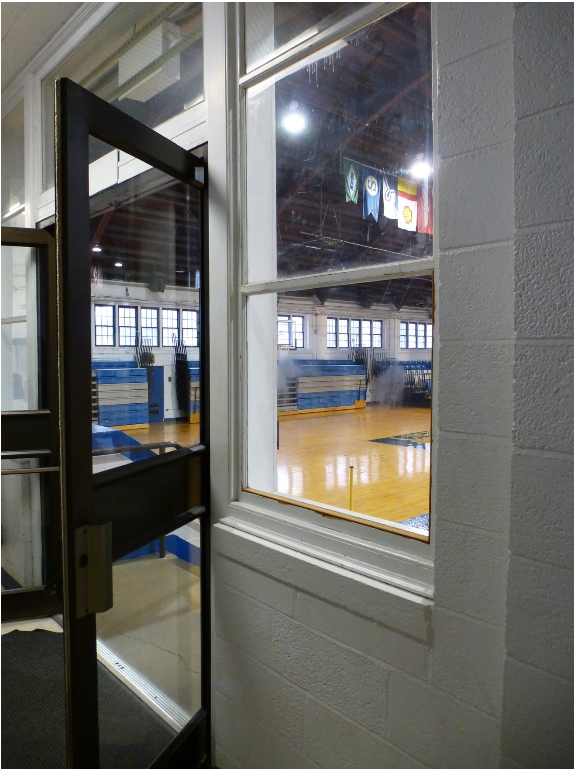
Figure 169. Original interior windows and doors between east vestibule and the drill hall at O'Hara Hall (ERDC-CERL, 2013).
