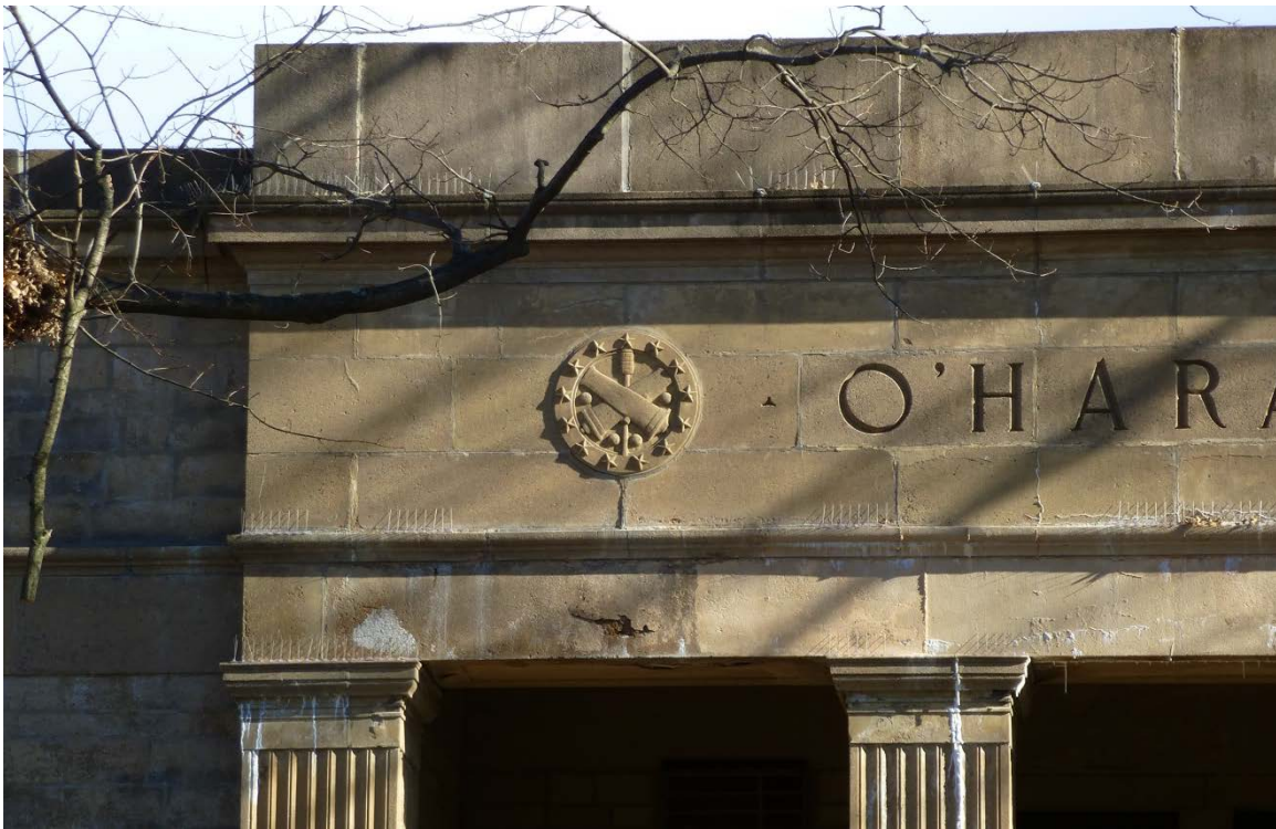
Figure 167. Detail of cast-stone elements on the portico at the west entrance of O'Hara Hall (ERDC-CERL, 2013).
