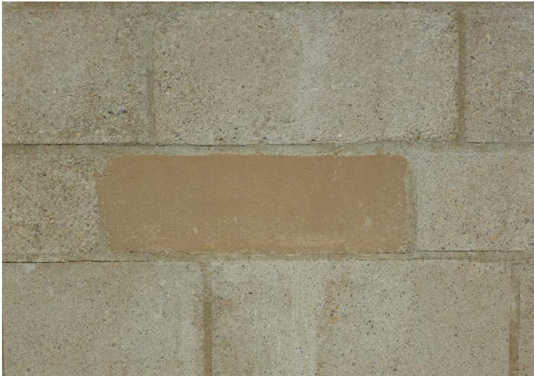
Figure 92. Detail of concrete block walls, showing distinctive stone-like pattern on these barracks (ERDC-CERL, 2013).
