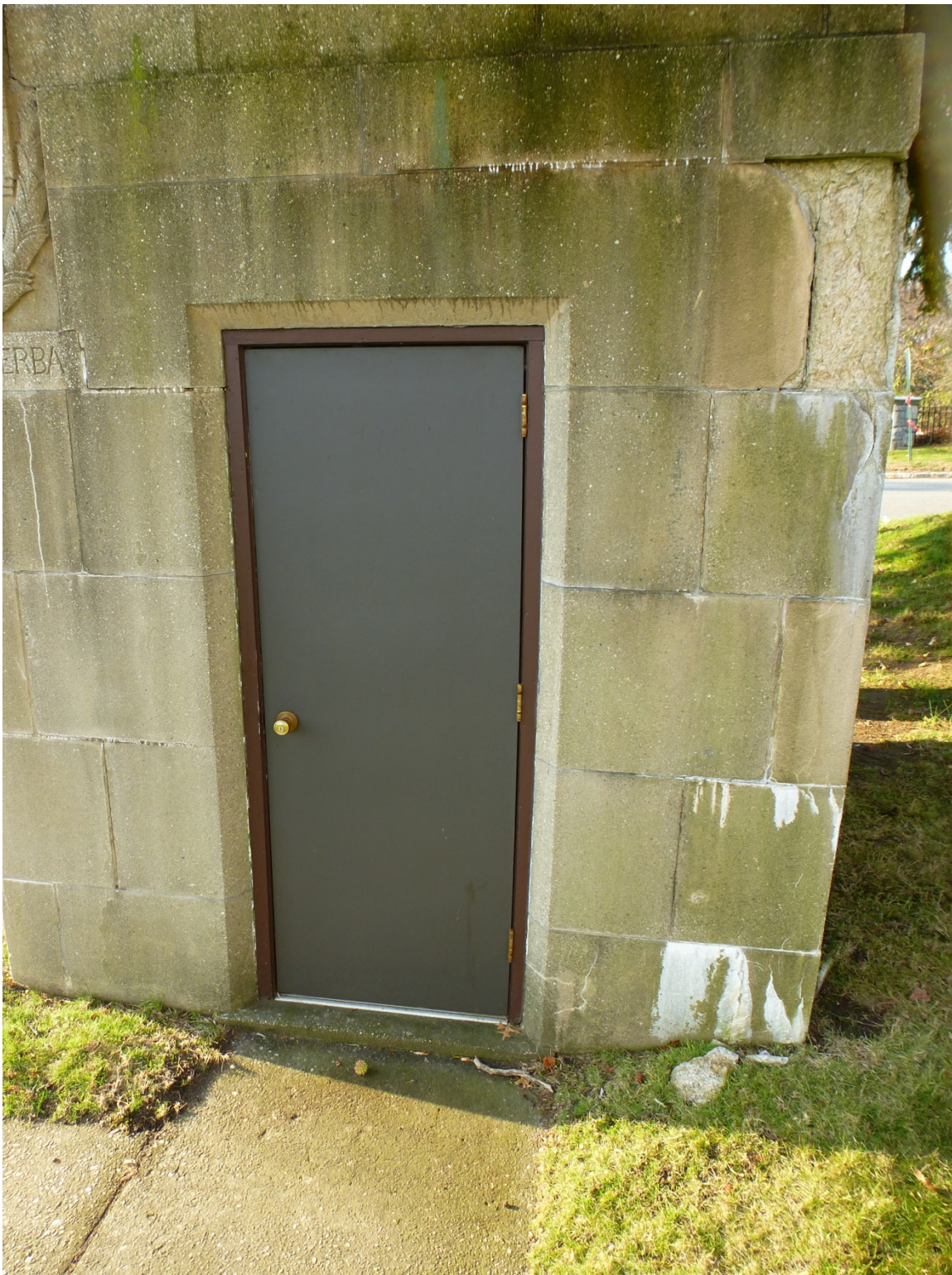
Figure 209. East façade of the Marvin Place Gate guard house on the north side of Steamboat Road, showing replacement door (ERDC-CERL, 2013).
