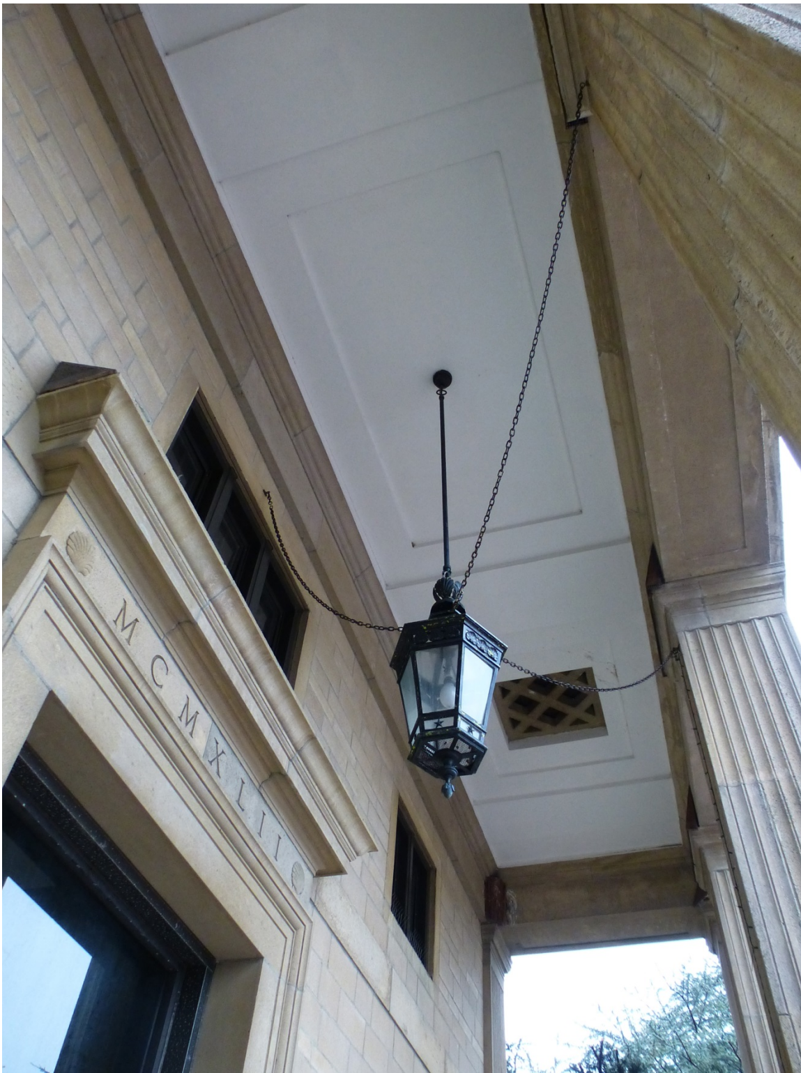
Figure 145. Original light fixture, ceiling, and cast-stone elements on the portico of Delano Hall (ERDC-CERL, 2013).
