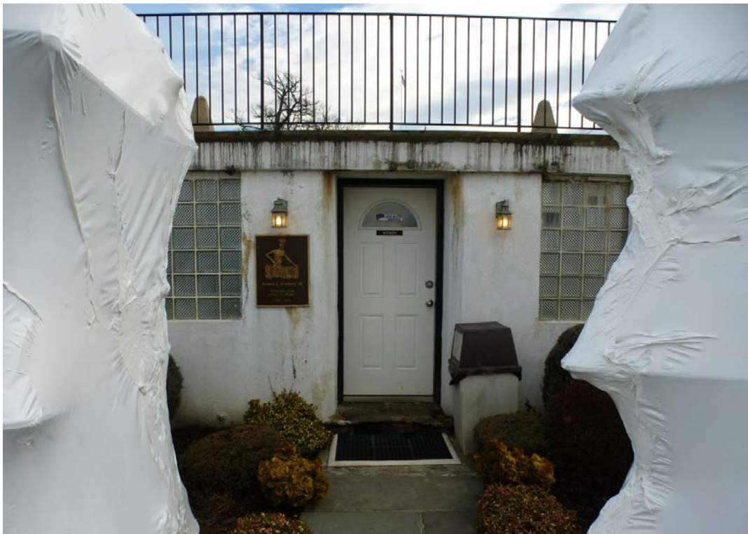
Figure 194. The replacement door into the women's shower near Eldridge Pool, shown flanked by wrapped training boats in foreground (ERDC-CERL, 2013).
