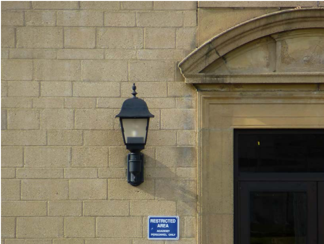
Figure 89. Cast-stone door surround and replacement light fixture on the west entrance to Palmer Hall (ERDC-CERL, 2013).
