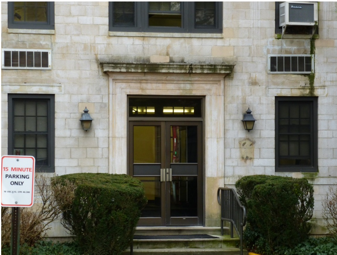
Figure 110. Windows, entrance doors, cast-stone surrounds, and exterior light fixtures on Furusetth Hall (ERDC-CERL, 2013).
