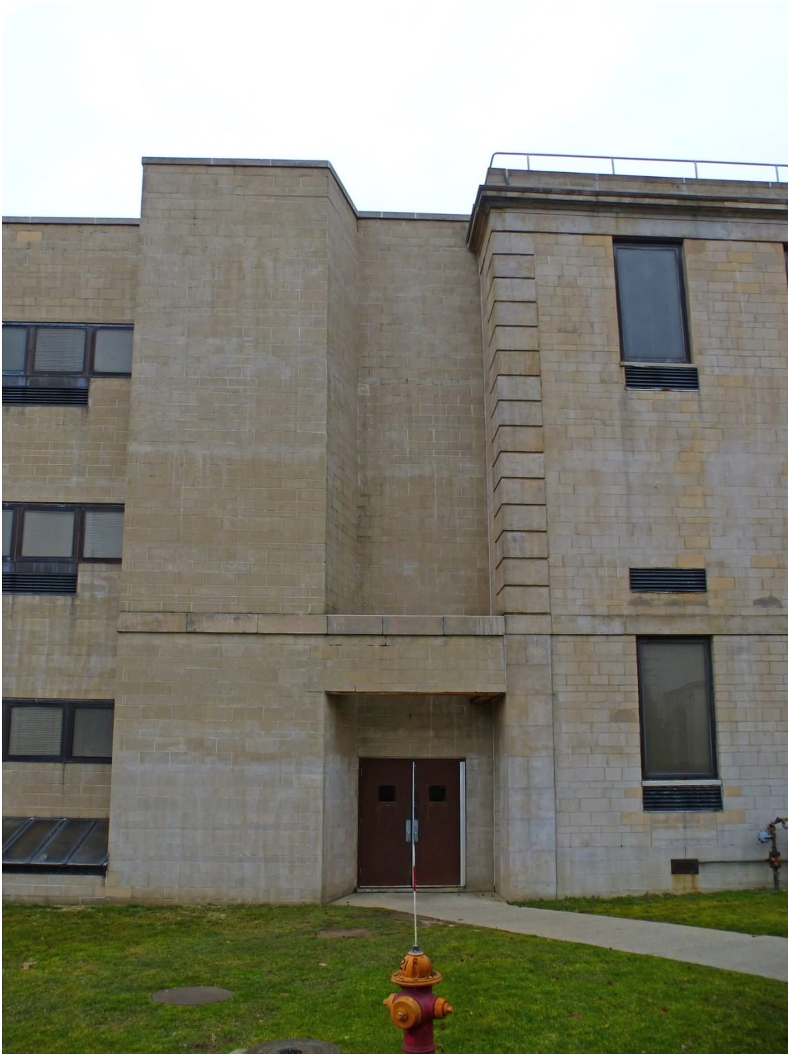
Figure 117. South façade of Gibbs Hall [left] and Fulton Hall [right], showing the transition between the two buildings (ERDC-CERL, 2013).
