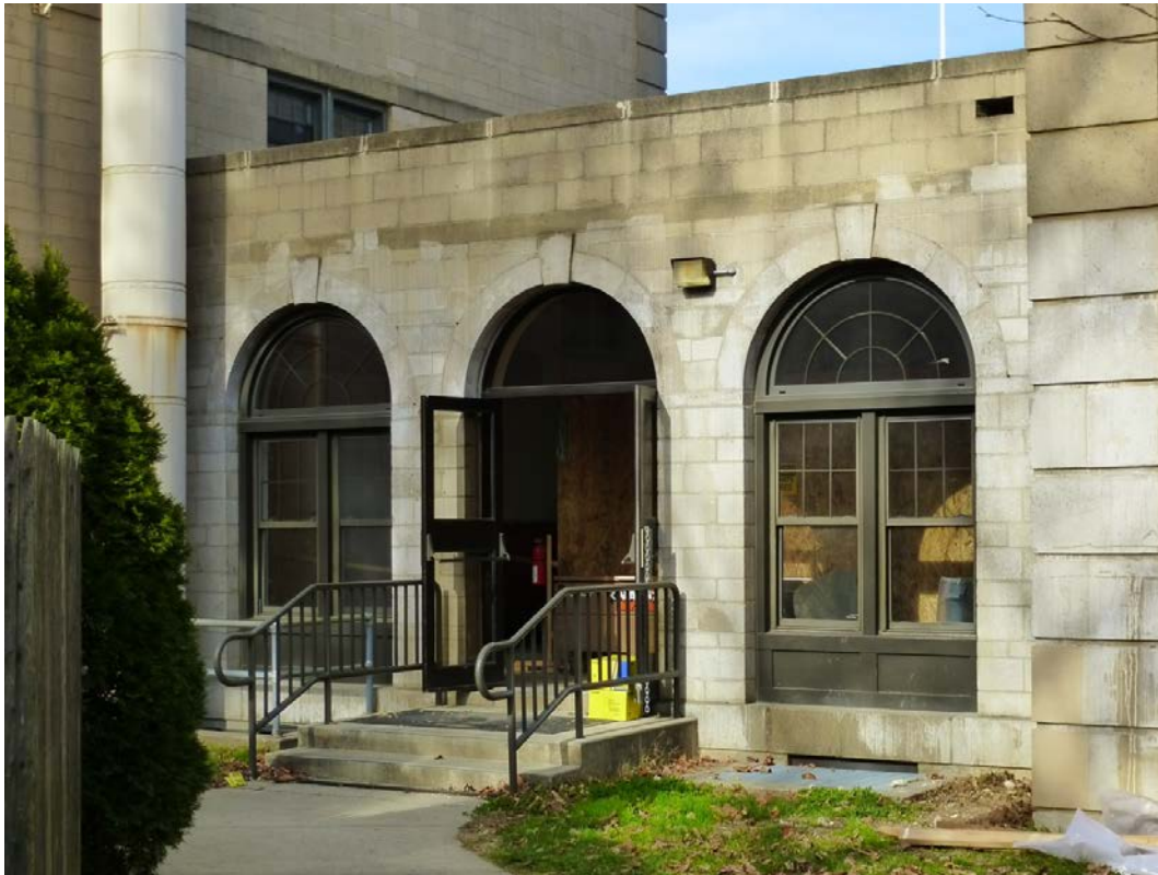
Figure 91. South façade of arcade that connects Rogers Hall to Cleveland Hall (ERDC-CERL, 2013).
