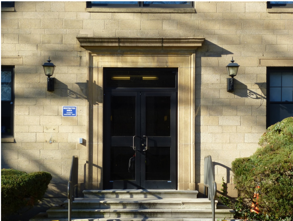
Figure 101. Detail of doorway on east façade of Barry Hall with nonhistoric doors (with original cast-stone surround), light fixtures, and railings (ERDC-CERL, 2013).
