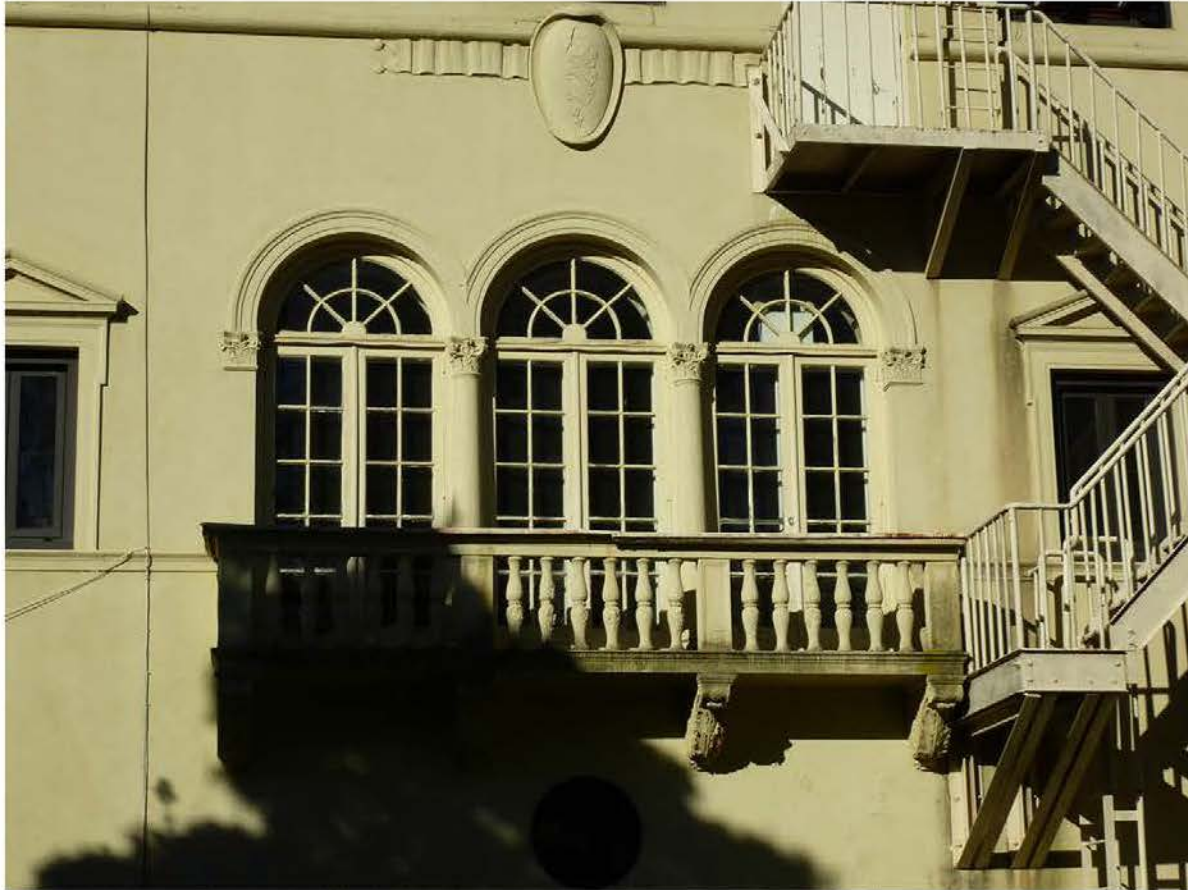
Photo 16. View to west of the French doors on the east facade that lead out from the second floor lounge.
