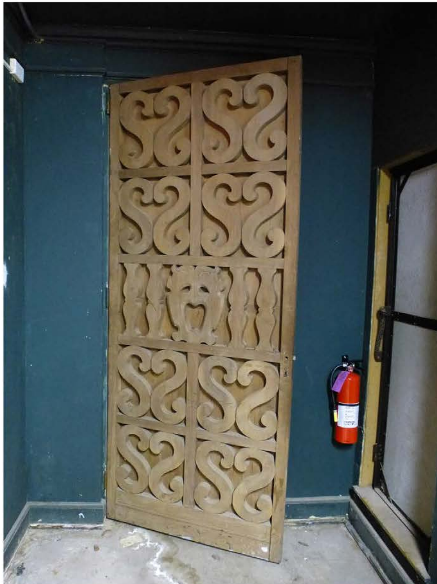
Photo 50. View to the south of a wood door in the movie theater in the basement of the music room addition.
