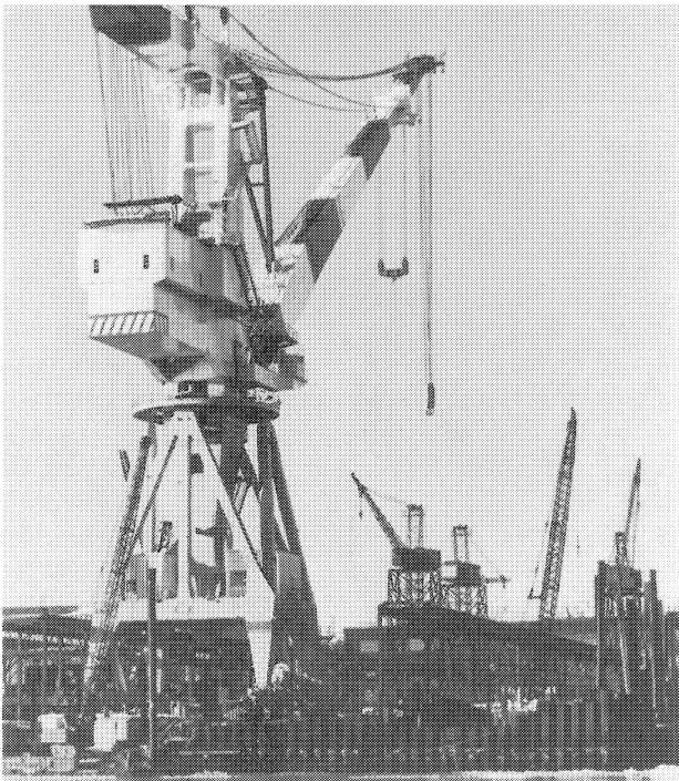
As part of modernization and expansion program, Bath Iron Works installed new 200-ton crane
