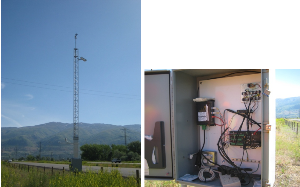
Figure 4.4 New Permanent ESS Installation
