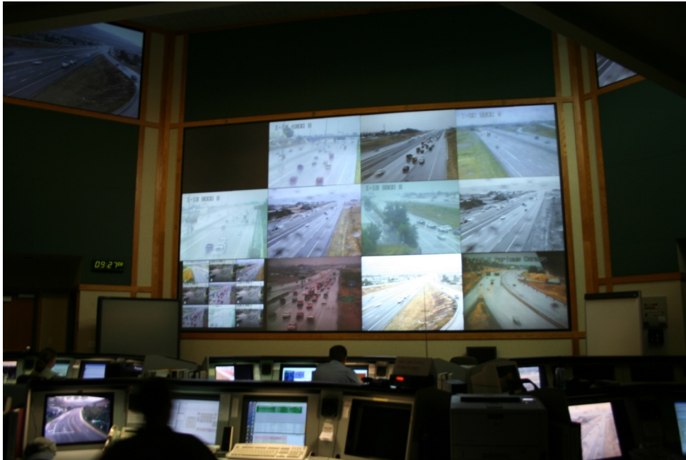
Figure 4.2 Utah DOT Traffic Operations Center Main Control Room
