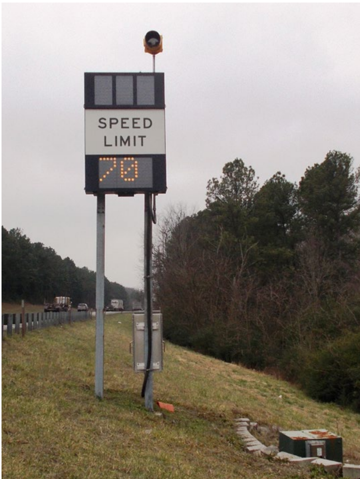
Figure 20. Variable speed limit sign in fog warning zone on I-75 near Cleveland, TN. Speed limit is reduced during periods of fog. (Source: Tennessee Department of Transportation)
