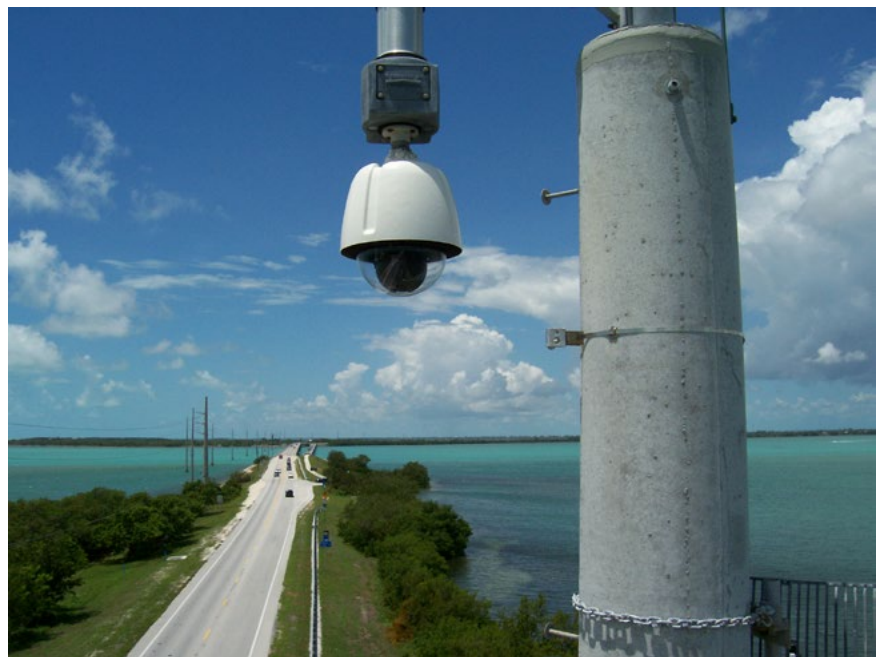
Figure 11. The use of checklists can help ensure the CCTV cameras and other ITS equipment effectively support operations. (Source: Florida Department of Transportation)
