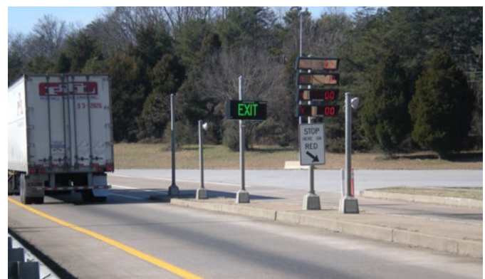
Figure 24. Weigh-in-motion station. (Source: Tennessee Department of Transportation)
