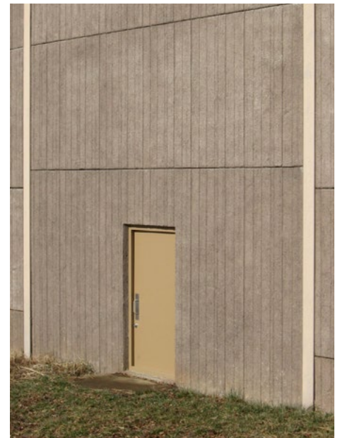
Figure 4. Access doors in noise walls like this one on Virginia State Route 267 can decrease incident response time. (Source: SAIC)
