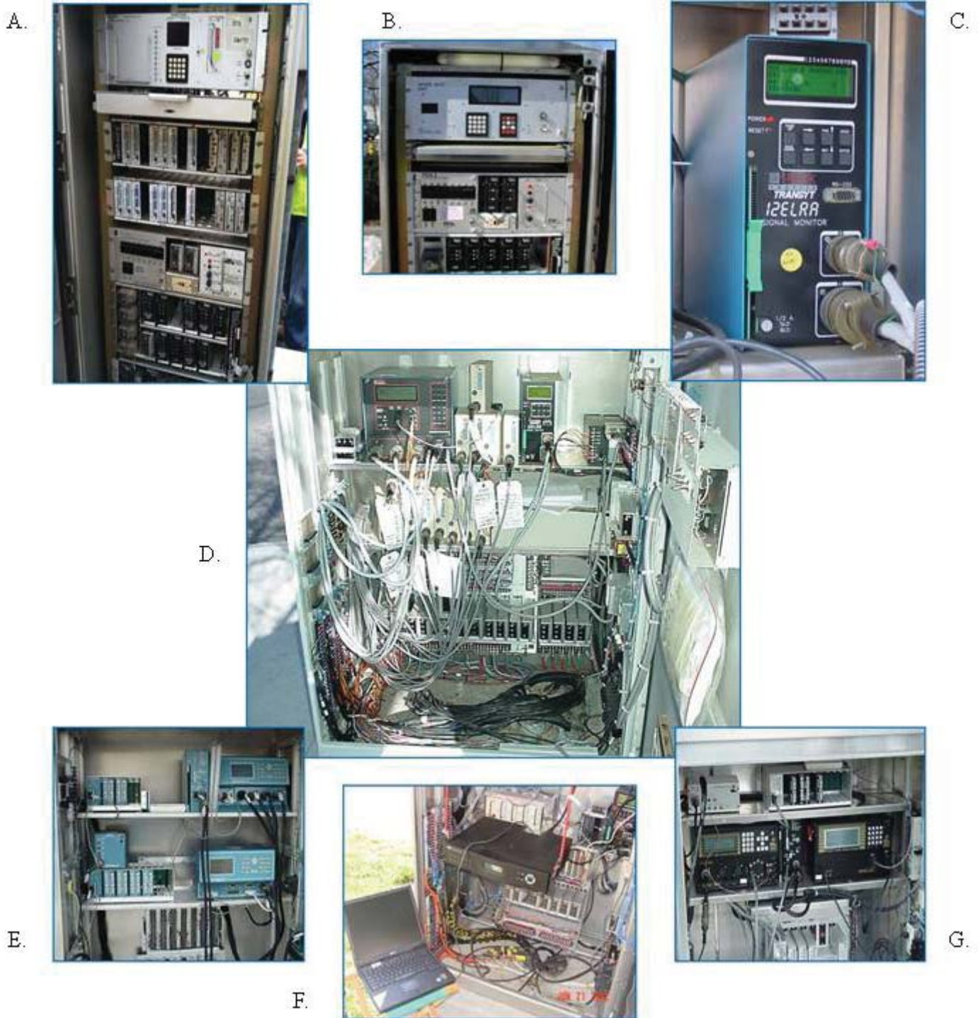
Figure 1: Field Examples of Highway Traffic Signal Controller Assemblies and Data Transfer Set-ups
