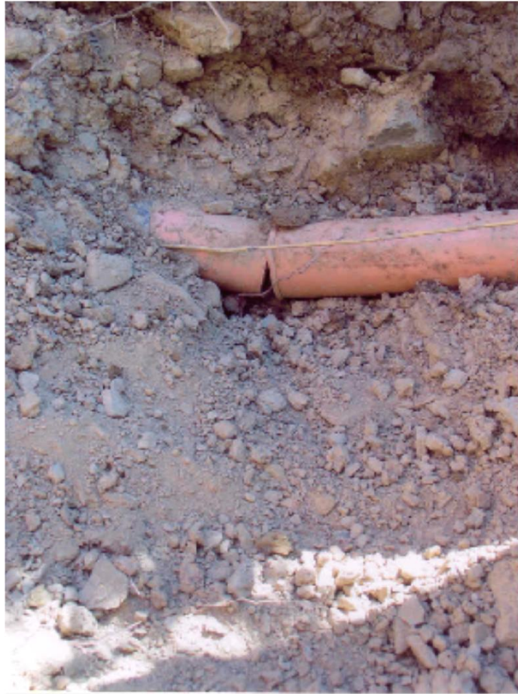
DuBois pipe failure
