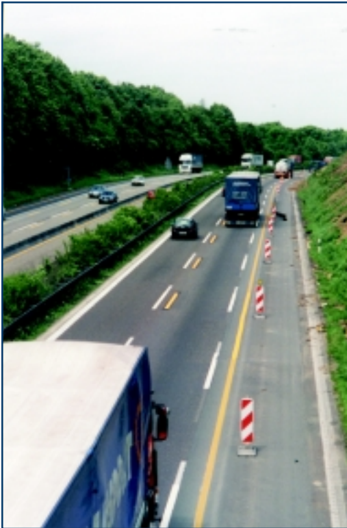
Figure 10. Both lanes have been narrowed in advance of a work zone in Germany, and trucks are restricted to the somewhat wider right lane.
