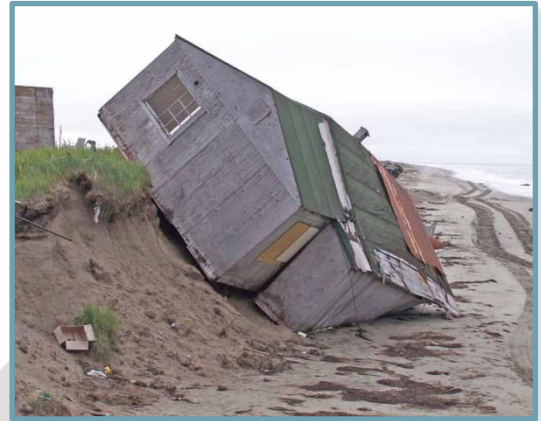
Coastal erosion in Shishmaref, near Bering Land Bridge National Preserve
