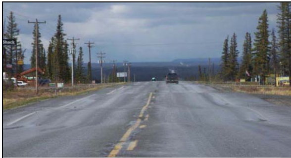
Glenn Highway, distress (ADOT&PF)
