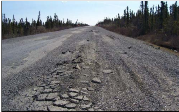
Dalton Highway, frost heaves (ADOT&PF)
