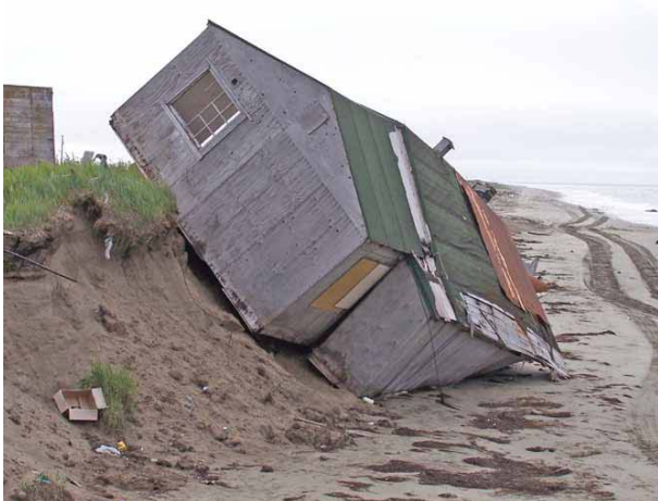
Storm erosion in Shismaref (NPS)
