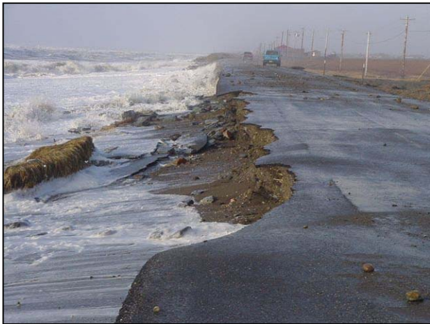
Coastal Erosion on Nome Council Road (ADOT&PF)
