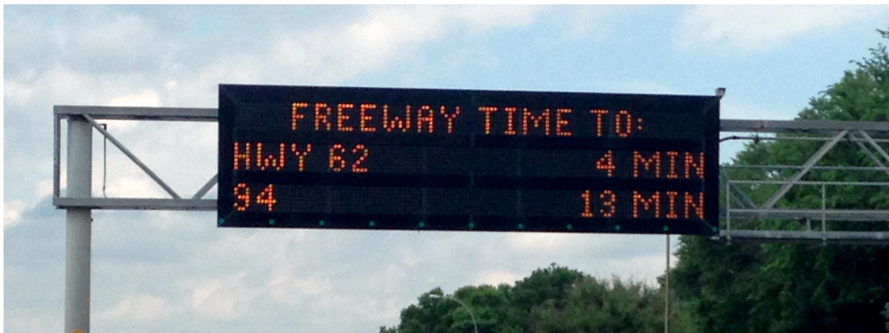
Figure 23. Photo. A TMC will have many technology and communications resources, such as the ability to display travel times captured from roadway detectors on a DMS.
