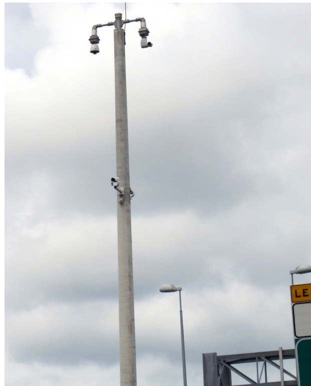
Figure 16. Photo. Managed lanes typically have extensive deployments of ITS equipment, such as these CCTV cameras.
