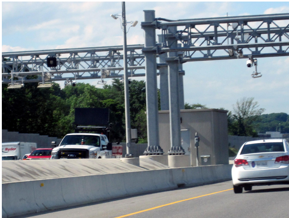
Figure 33. Photo. Pre-positioned service vehicles or service vehicles on a roving patrol can monitor the managed lanes and provide quick response if an incident occurs.
