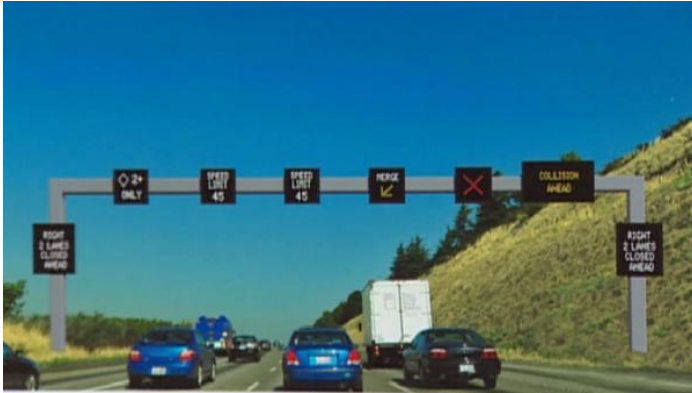
Figure 22: Variable Speed Limit Sign with Lane Controls, Seattle, Washington (courtesy Washington State Department of Transportation)
