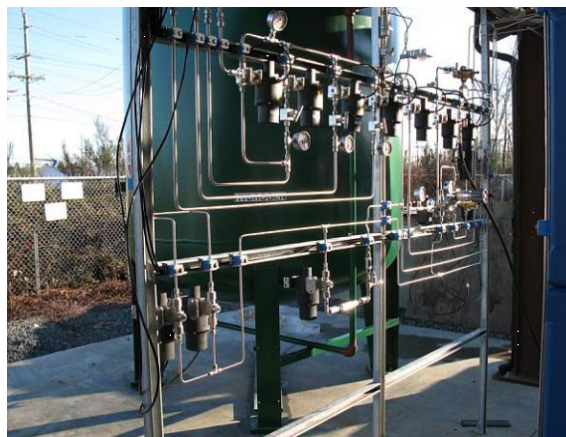
Figure 7. Powertech Labs SAE J2579 Pneumatic Test Facility Inlet Flow Control Panel.
