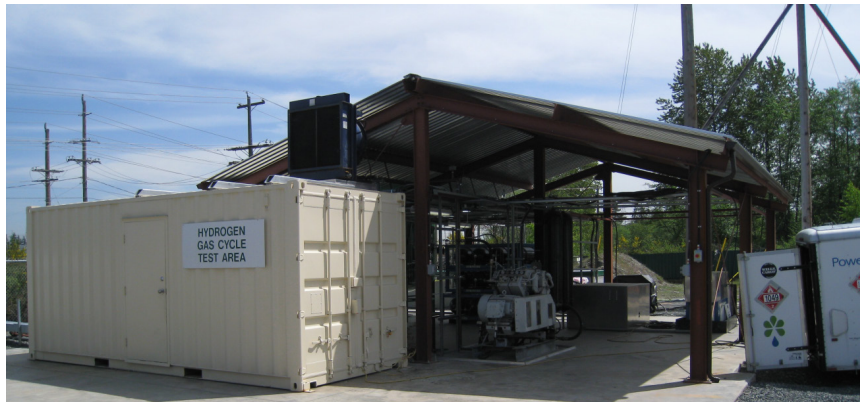
Figure 6. Powertech Labs SAE J2579 Pneumatic Test Facility.
