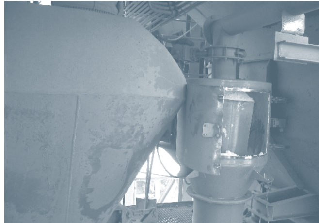
Figure 26. Batch hopper for batch plant.
