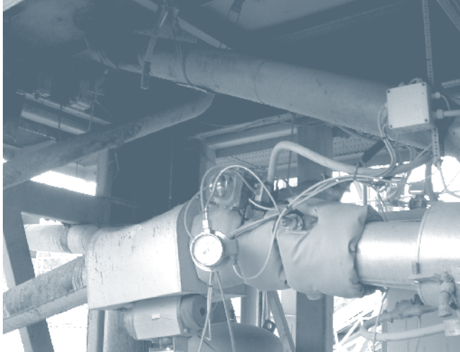
Figure 33. Asphalt line, expansion chamber, controls, and transfer pipe for foaming hard asphalt.
