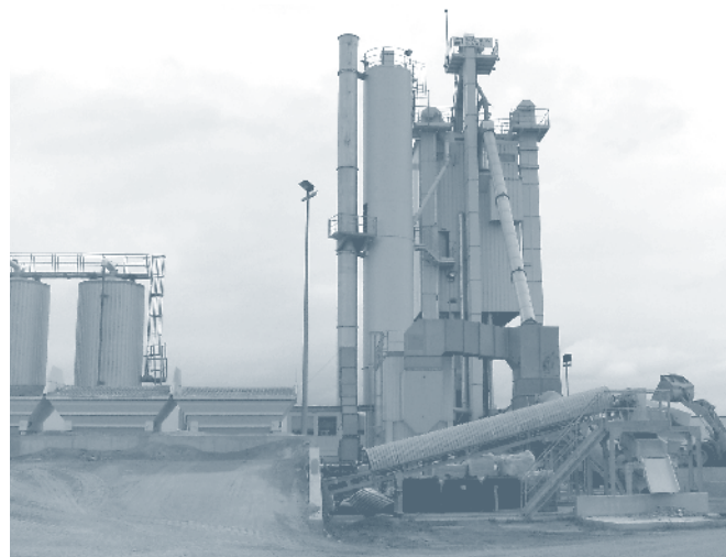
Figure 15. EIFFAGE Travaux Publics batch plant in France.
