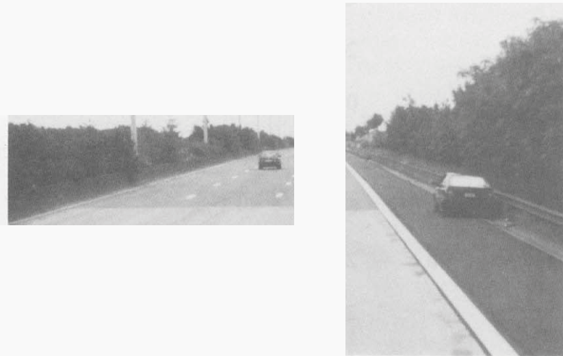
Figure 3.15 20-year-old CRCP in Belgium containing 0.85 percent reinforcement, AC interlayer, lean concrete base and a granular subbase. (Note that a portion was diamond ground to reduce noise emission of the original transverse tining).
