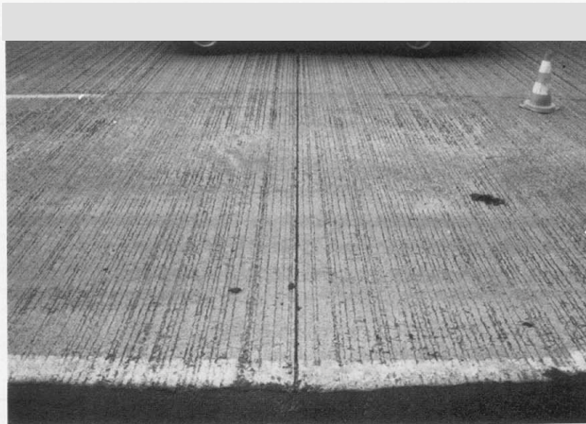
Figure 3.18 Surface and transverse tining of fiber-reinforced concrete overlay of an AC pavement in Belgium.
