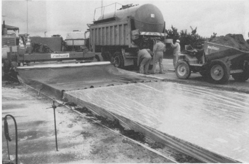
Figure 3.16 Polyethylene sheeting placed over concrete surface after retarder has been sprayed (Robuco process). (4)
