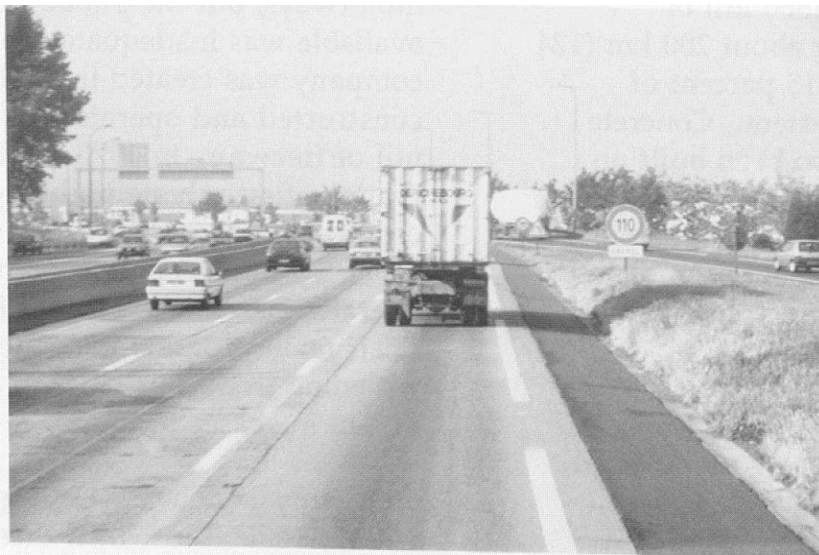
Figure 3.1 Thirty-year-old JPCP section of the A6 south of Paris. (Note added lane with widened edge.)
