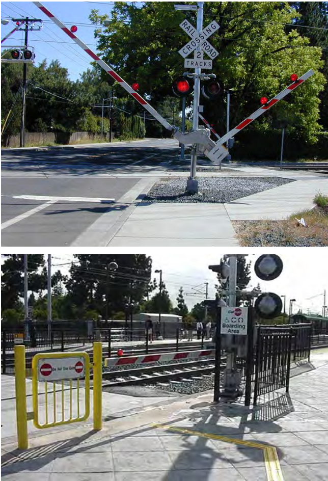
Figure 76. Pedestrian Automatic Gate Examples
