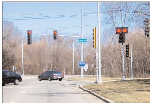
Figure 3-10. Supplemental Signal for an Intersection in the Middle of a Reverse Curve.
