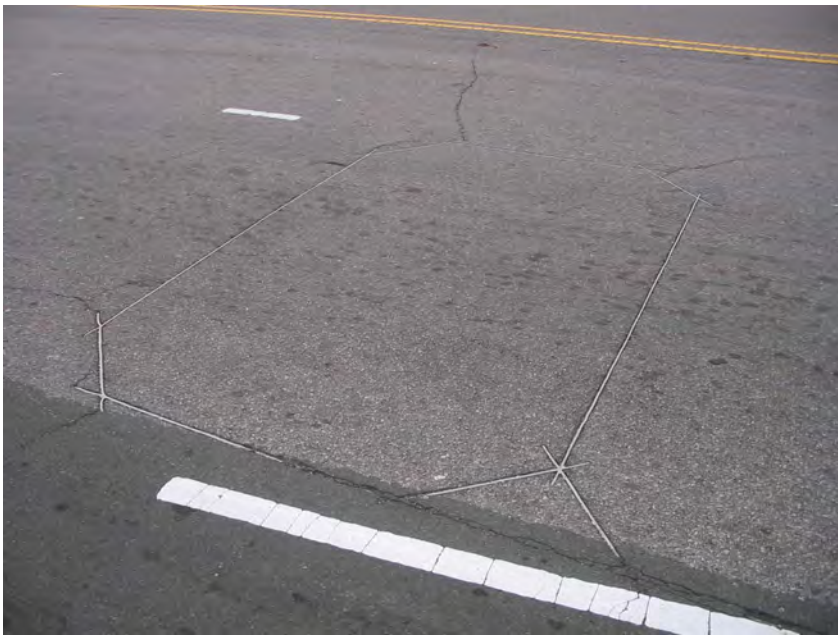
Figure 3-2. Vehicle detector loop in pavement.
