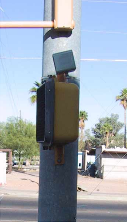
Figure 1-2. Pedhead-mounted APS. The speaker is mounted on top of the pedestrian signal head.
