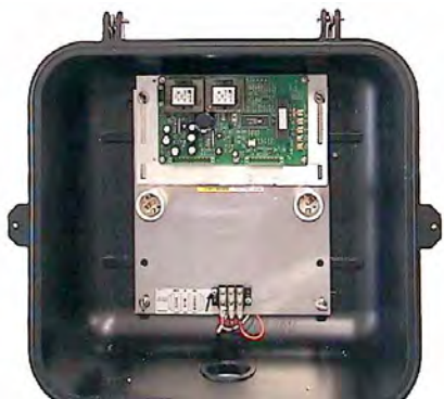
Figure 6-20. Controller board mounted behind 18-in. pedestrian signal head.
