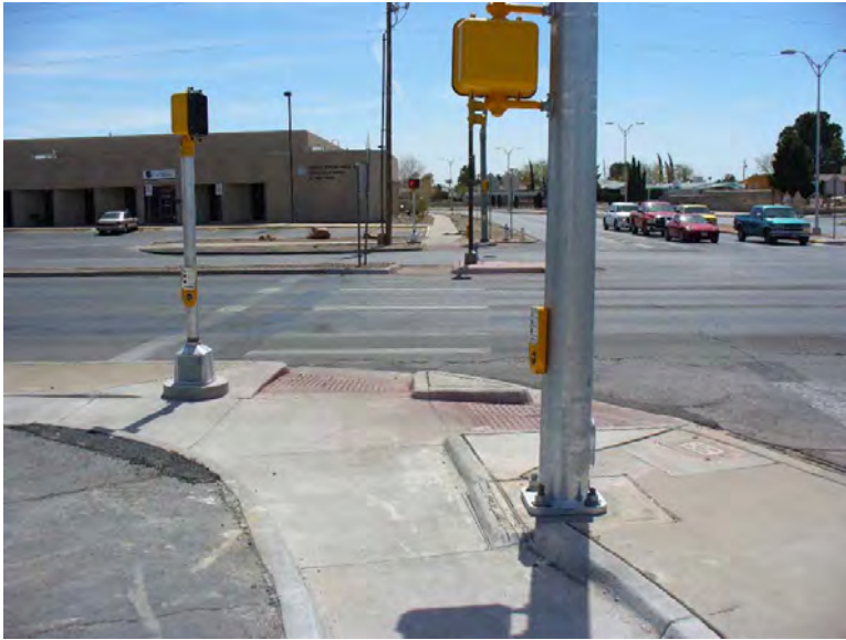
Figure 7-15. APS pushbuttons installed incorrectly.
