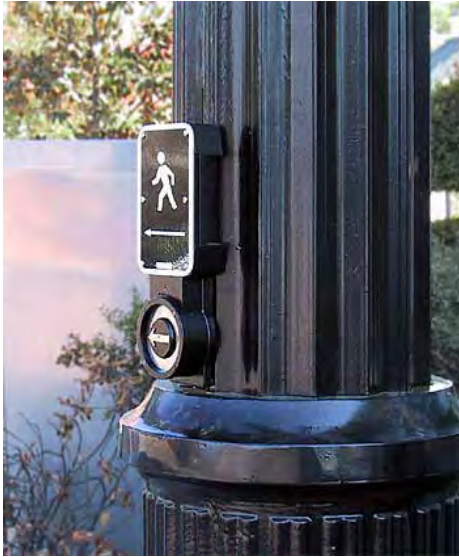
Figure 7-7. A misaligned APS, with the arrow pointing into the bushes.
