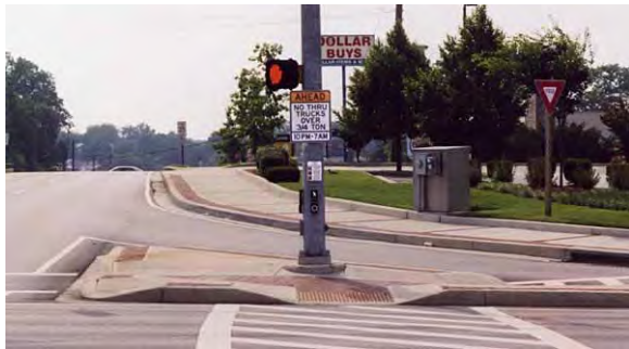
Figure 9-12. Two APSs are mounted on the existing pole on this island.
