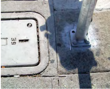
Figure 6-30. Stub pole installed near sidewalk signal box simplifies wiring and locates ped pushbutton by the crosswalk
