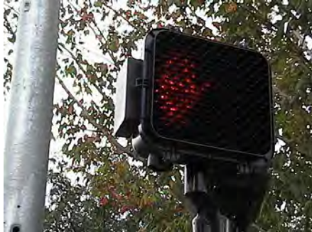
Figure 6-19. External mount for controller board is visible on the left side of the pedestrian signal head.
