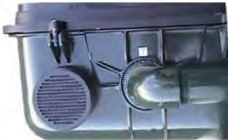
Figure B-4. BBU, showing speaker mounted on bottom of pedestrian signal head.
