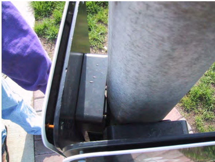
Figure 7-14. Incorrect installation of two APSs on a single pole (no vibratory insulation).
