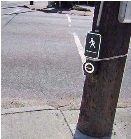
Figure 7-13. The APS was temporarily replaced on the pole, but the tactile arrow points to the center of the intersection, rather than being aligned with the direction of travel on the crosswalk.
