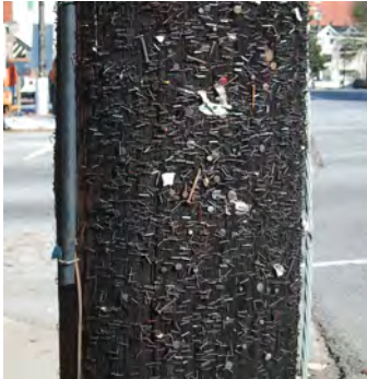
Figure 6-26. Wooden pole with nails and staples that are a source of concern.
