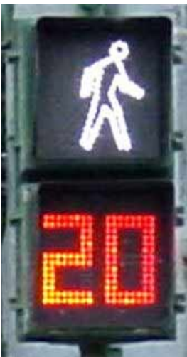
Figure 3-9. Incorrect countdown display, showing countdown during the “Walk” interval.
