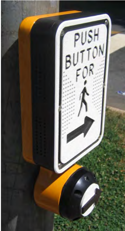
Figure 4-2. This accessible pedestrian signal has a high-contrast, raised tactile arrow on the pushbutton and a high-contrast, recessed tactile arrow on the sign above the button.
