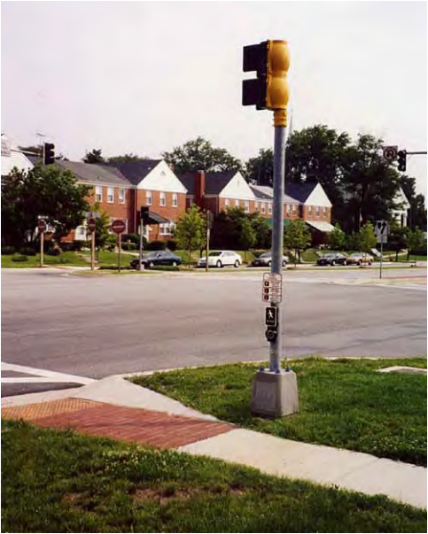
Figure 9-14 APS installed on pedestrian signal pole.
