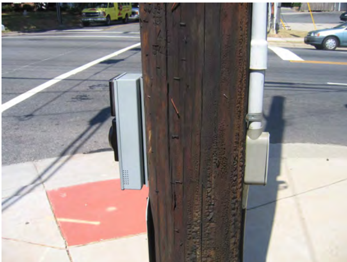
Figure 6-25. This APS is mounted on a wooden pole by drilling a hole through the pole and running wires through the back of the device.
