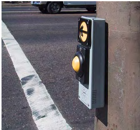
Figure 9-4. Vibrawalk pushbutton installed in Portland includes a locator tone. The arrow vibrates during the walk interval and a “Walk” indication is provided from the pushbutton or speaker mounted on the pedhead.
