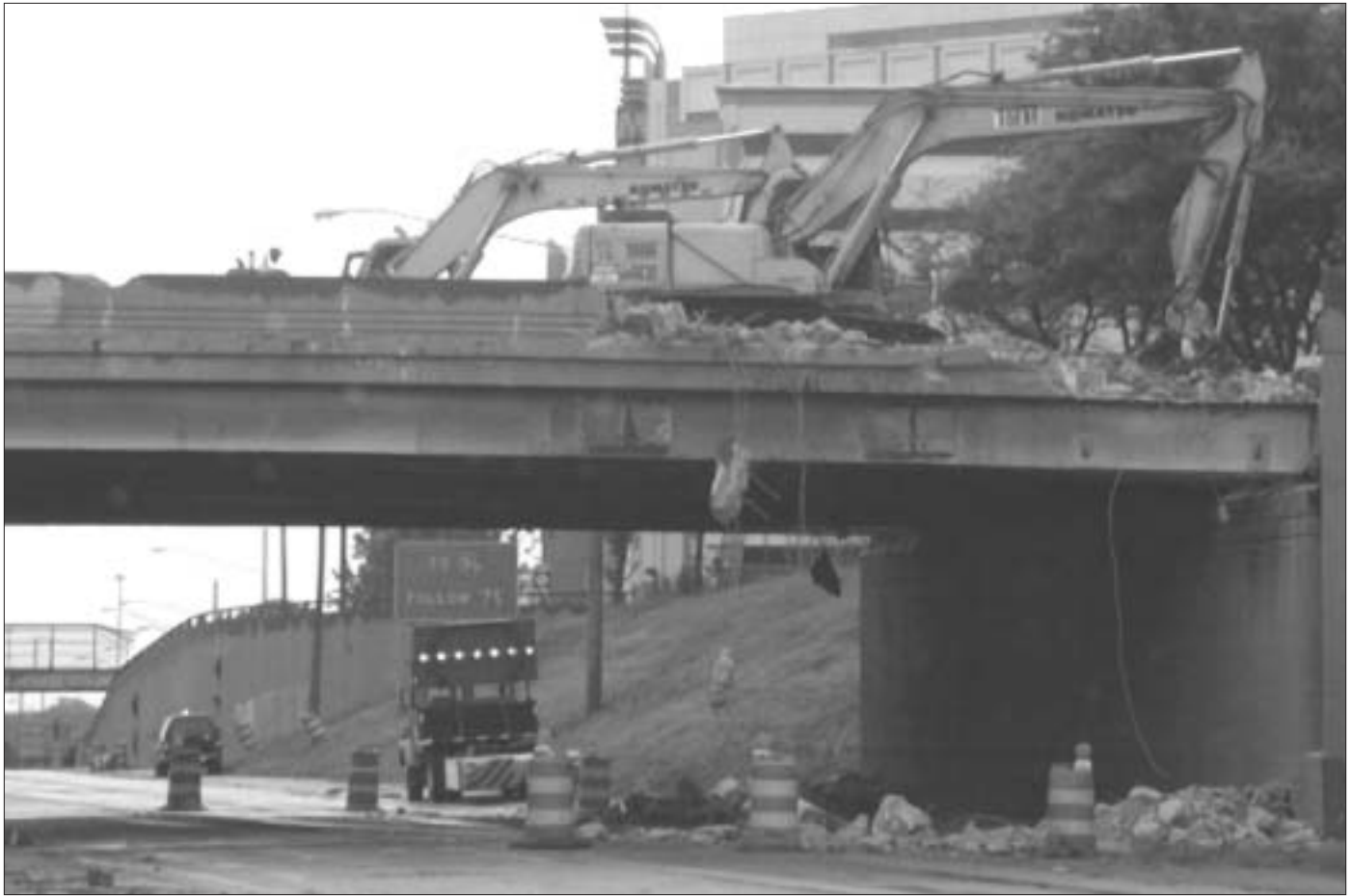
Figure 2 – The requirement for significant bridge repairs made full road closure an attractive option during the M-10 reconstruction
