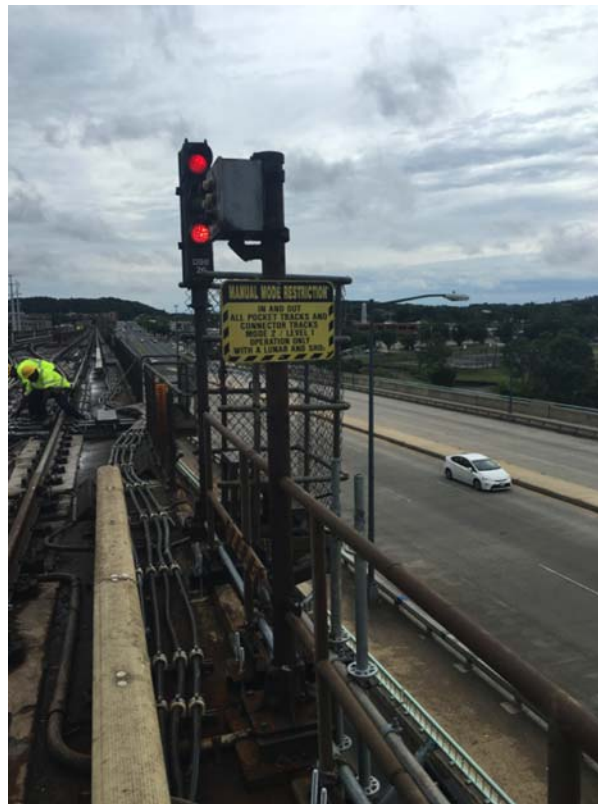
Figure 8: Sign installed near D&G Junction
