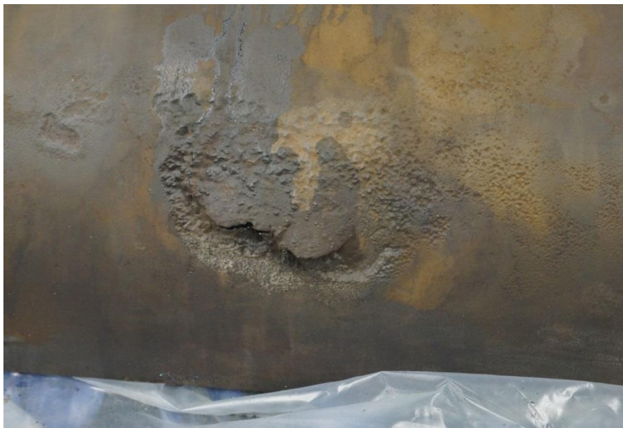
Pipe External Surface at the Line 901 Failure Site
