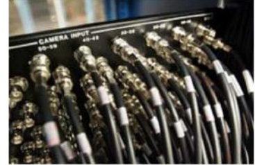
Cabling used for video processing in a TMC.
