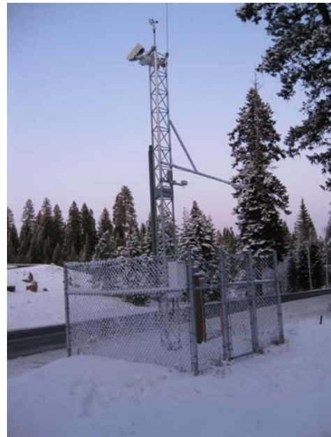
Figure ID-1. RWIS installation at Goose Creek Summit on State Highway 55 in central Idaho.
