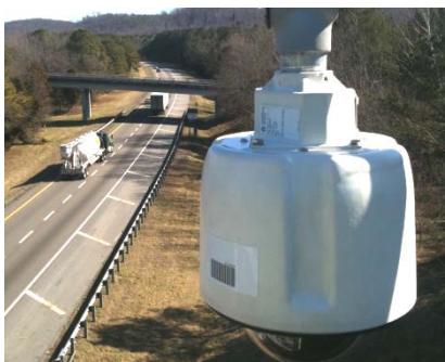
Figure TN-2. CCTV camera.
