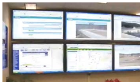
Figure VT-1. Traffic operations center.
