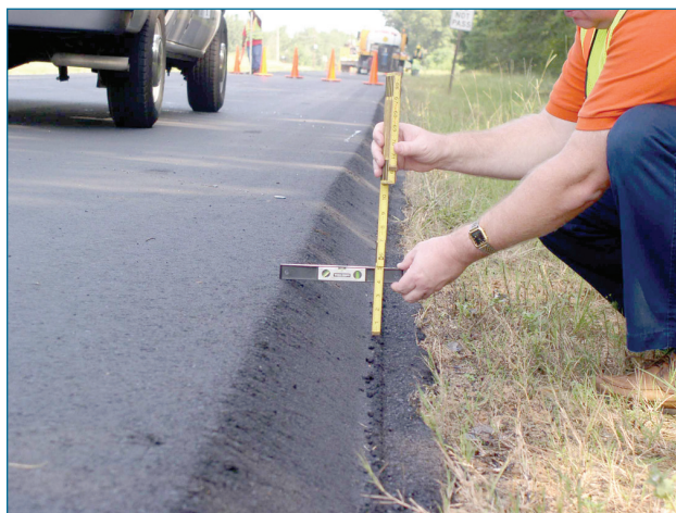
An inspector measures the angle of the tapered pavement edge of a newly paved road. SafetyEdge SM is one of the most successful innovations implemented by the Every Day Counts initiative, and the EDC marketing team was one of the first to complete NHI's Leap Not Creep training.
