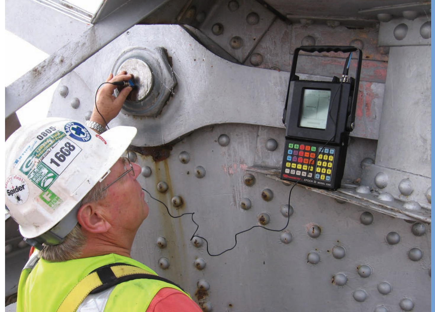
This inspector is conducting ultrasonic testing on a steel bridge component. Credit: Phil Fish, Fish & Associates, Inc.
