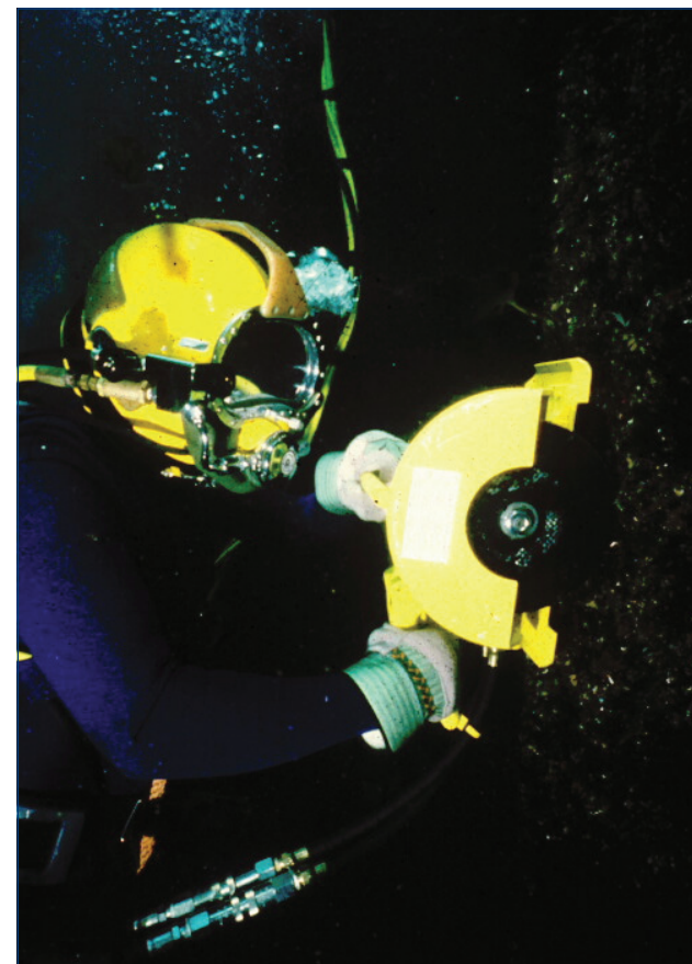
A diver makes underwater bridge repairs with a hydraulically driven circular cut-off saw.
