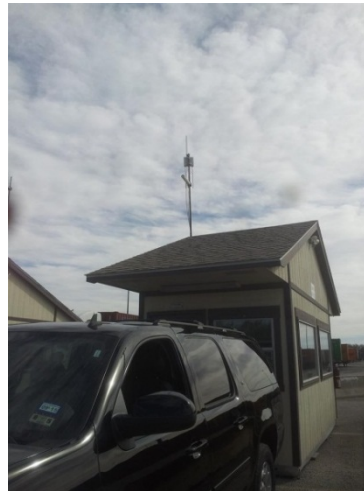
DSRC RSU (Long view)
