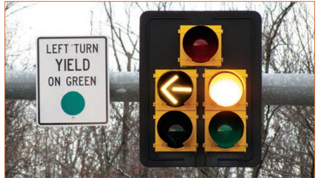
NHI developed four new courses designed to help practitioners improve the timing design, operation, and maintenance of traffic signals like these.
