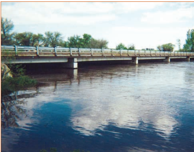
Flood waters are lapping at the bottoms of this bridge's pier caps. Instructors show this photo, along with floodplain maps and other hydraulic data, in one of the case studies for course 135090.
