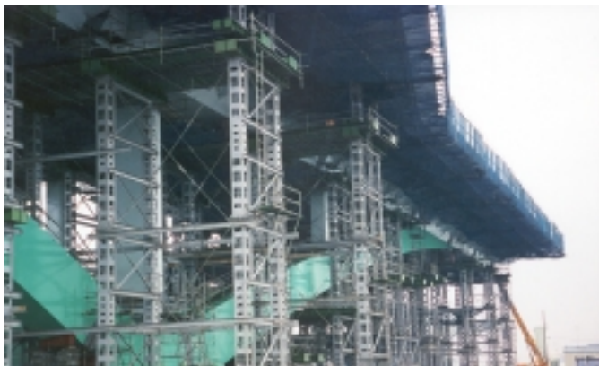
Figure 3. Yokogawa Bridge Corp.'s Osaka plant wharf containing the 2000-ton, 115.1-m segment for North Kyushu Airport Connection Bridge in Japan.
