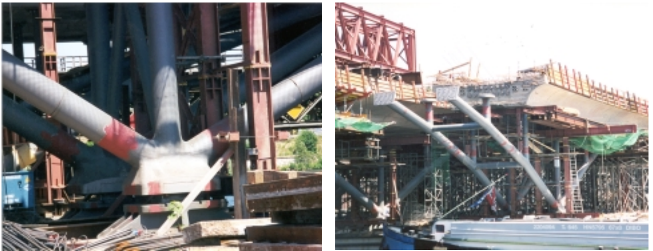
Figure 22. Large-cast steel bearing connections and tubular support structure, with cast steel nodes, of the Humboldthafen Rail Bridge in Germany.
