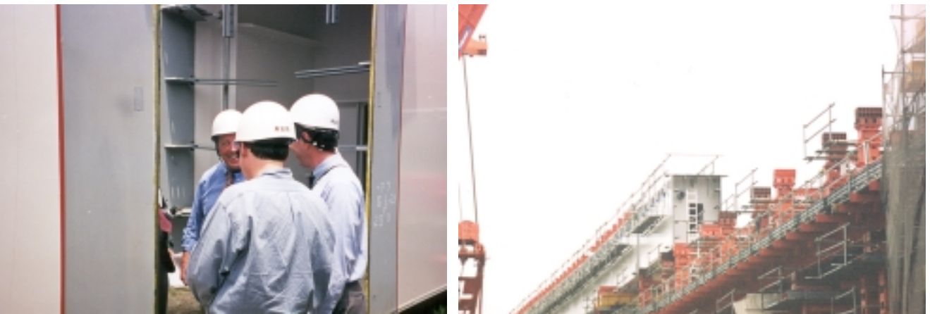
Figure 12. Fabricated box sections stored on site at Inabe River Bridge in Japan.
