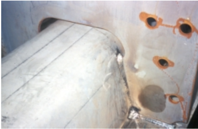
Figure 39. Typical weld intersection on deck section in Japan.
