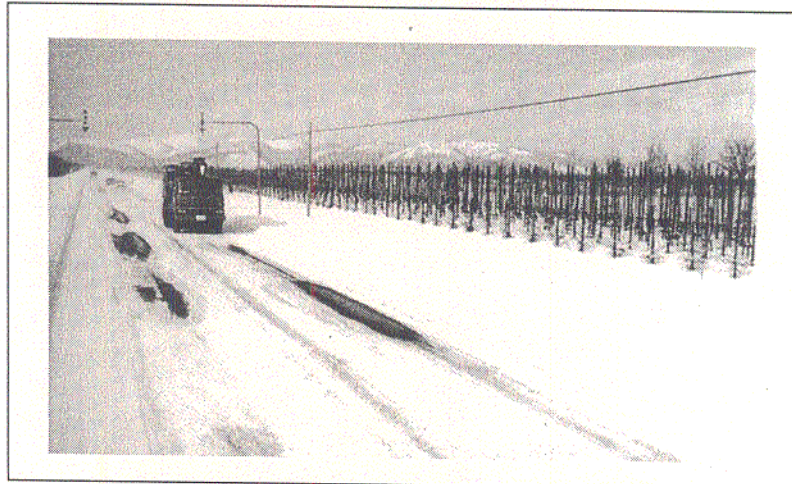
2. Ordinary National Highway Number 40, Nakagawacho, Kokufu. Highway snowbreak forest under construction. (Hokkaido Development Department)
