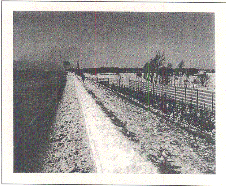
4. Hokkaido Jukan Highway, Sapporo-Iwamizawa. Highway snowbreak forest under construction. (Japan Highway Public Corporation, Sapporo Construction Department)
