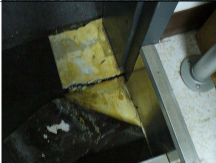
Building 2767. The floor in the computer room has significant cracks.
