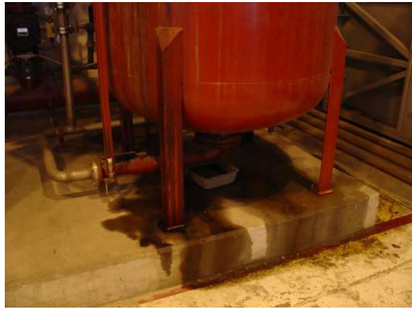
Figure 10.-Hangar 51 leaking AFFF storage tank.
