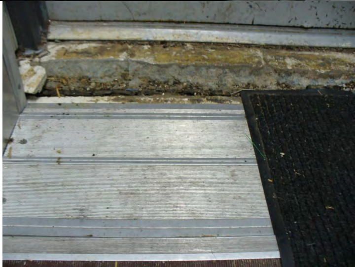
Building 2767. The floor near the hallway entrance sank over an inch and is cracked.
