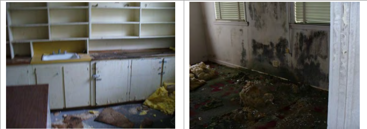
Figure 1.-NASCC, Building 5 was condemned due to poor condition and mold. The building is vacant with no funding available for demolition.
