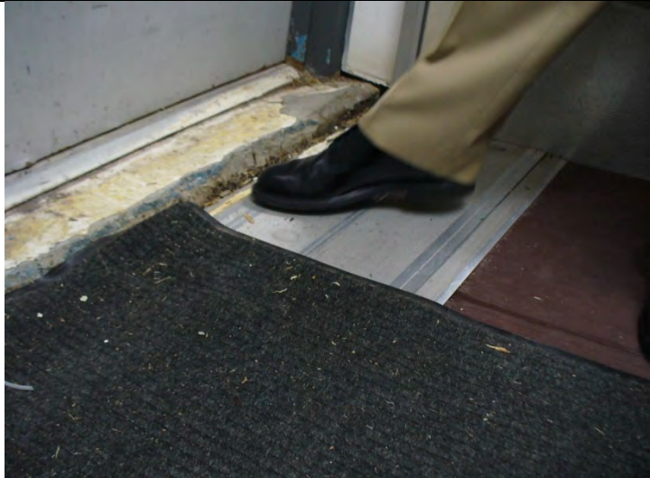
Building 2767. The floor in the computer room sank over an inch and cracked the slab near the exit door.
