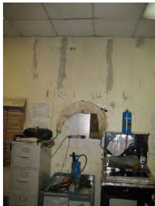
Figure 7.-Poor condition of work area.
