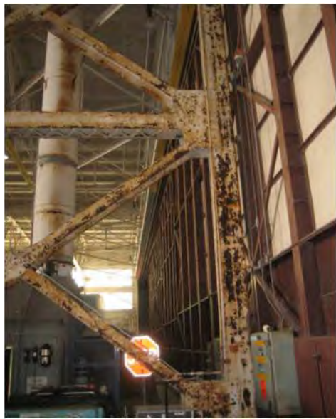
Figure 2.-Rusted Structural Beams
