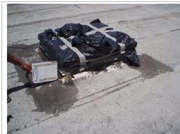
Figure 4.-Damaged Roof Vent
