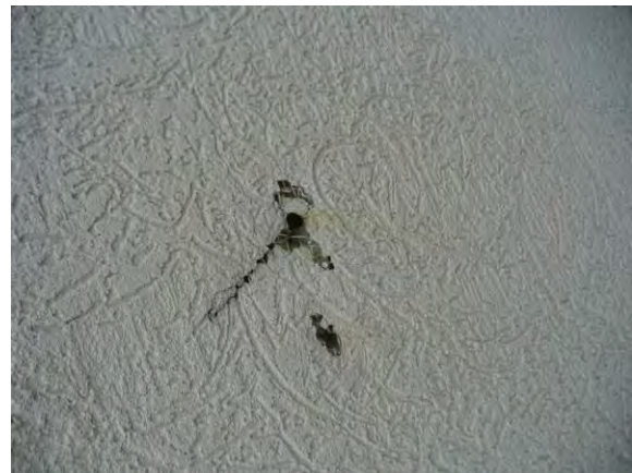
Figure 12.-Building 2 EIFS punctures allowing moisture penetration.
