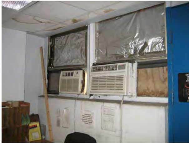
Figure 5.-Poor condition of shops spaces. Window air conditioning units needed to cool space.
