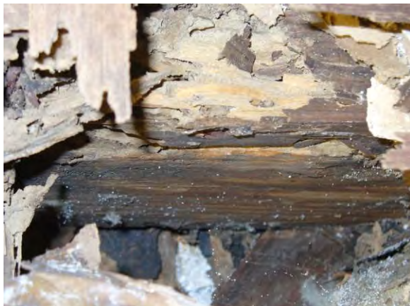
Figure 11.-Building 2 exterior wall studs rot due to moisture infiltration.
