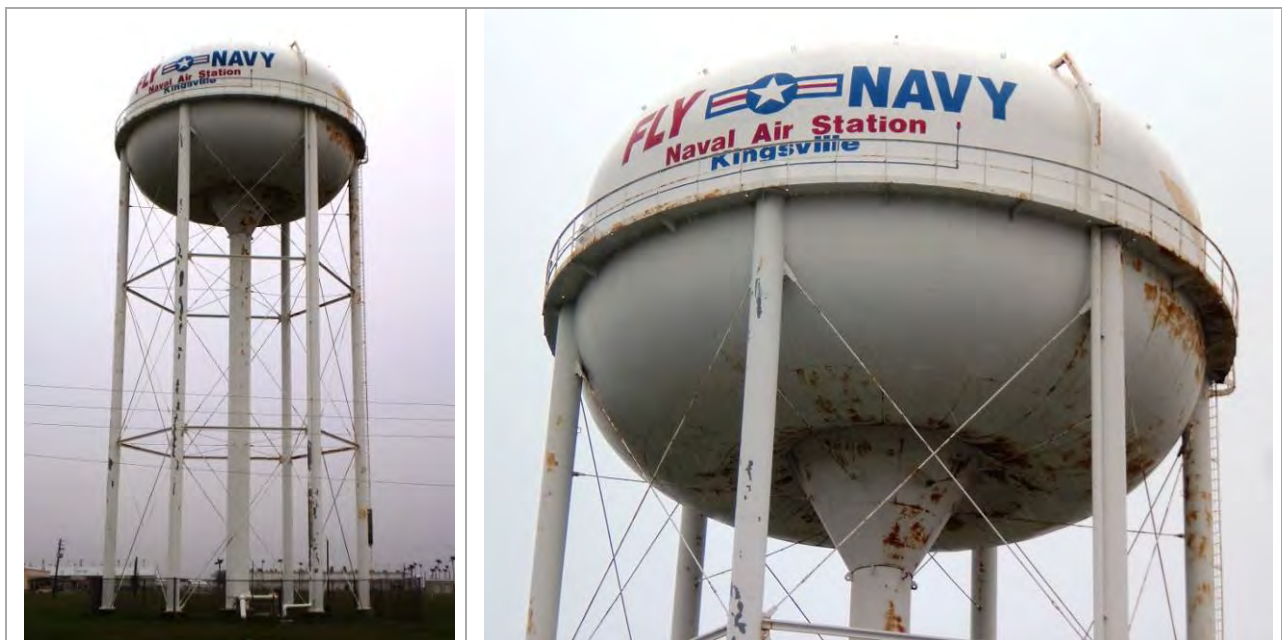
Figure 24.-Corroding 500K gallon elevated water storage tank at NASK.
