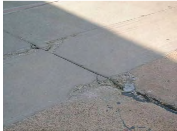
Figure 6.-Cracked and Failing Pavement
