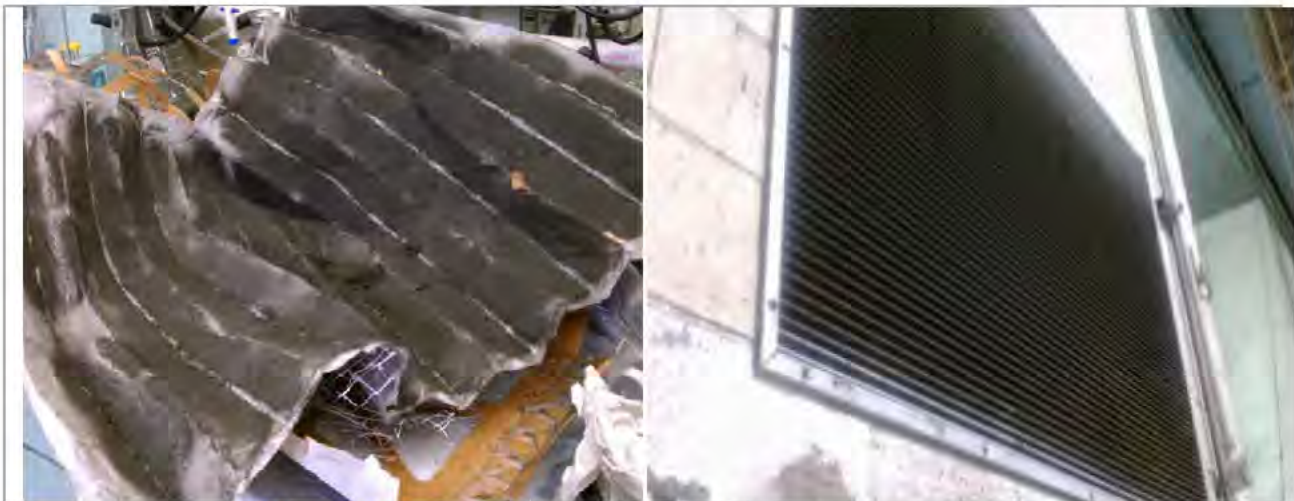
Figure 17.-Contaminated HVAC air filters from Building 1808.
