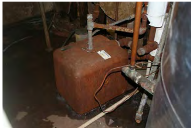
Figure 8.-Steam condenser needing replacement.
