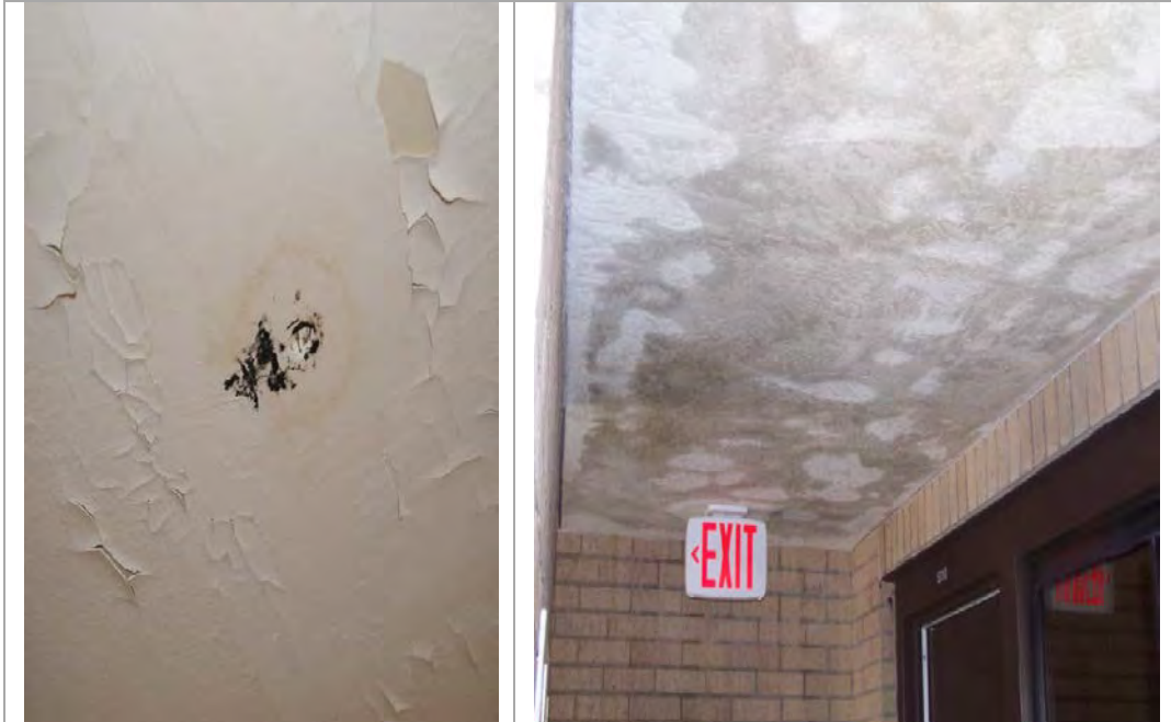
Figure 25. - Mold and water damage at NTTC barracks, Lackland AFB.
