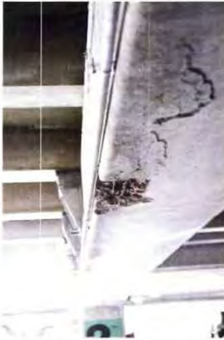
Figure 1: NMIC Garage - Main support beam on 2nd deck in state of failure
