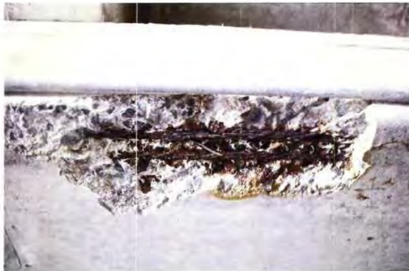
Figure 2: NMIC Garage - Detail look at compromised rebar/pre-stressed bar (2nd deck main support beam)
