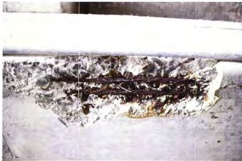
Figure 2: NMIC Garage - Detailed look at compromised rebar/pre-stressed bar (2nd deck main support beam)
