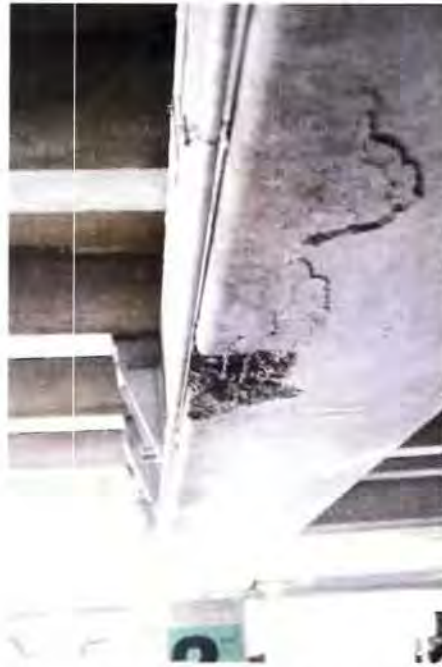
Figure 1: NMIC Garage - Main support beam on 2nd deck in state of failure
