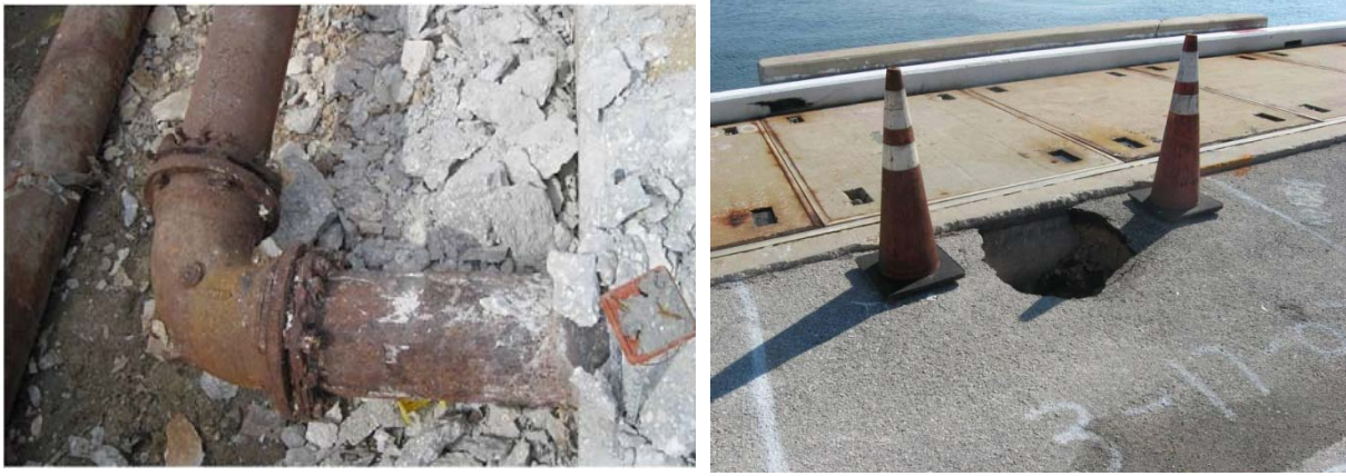
Figure 1- Deterioration at the Wharfs on NS Mayport
