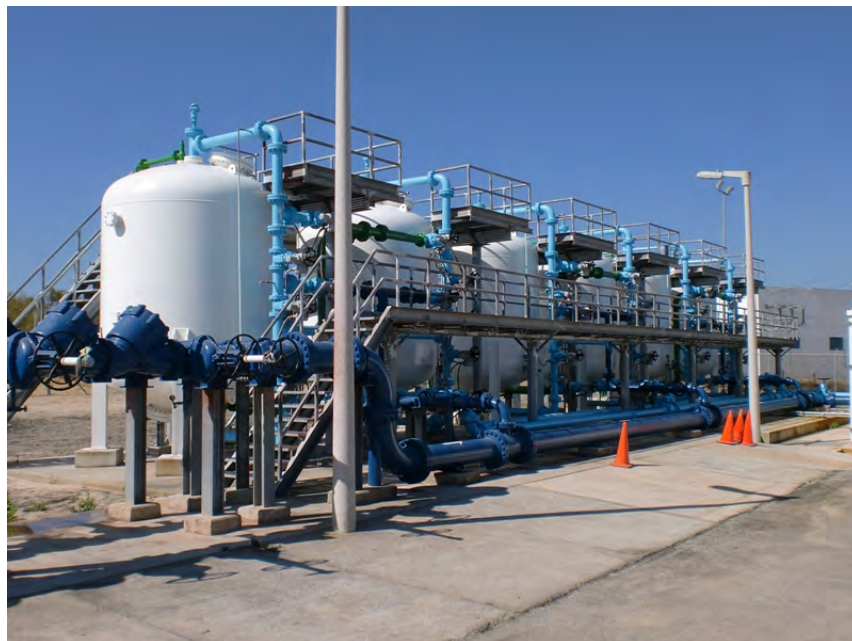
Figure 9 – Granular Activated Carbon Treatment System at Naval Station Rota
