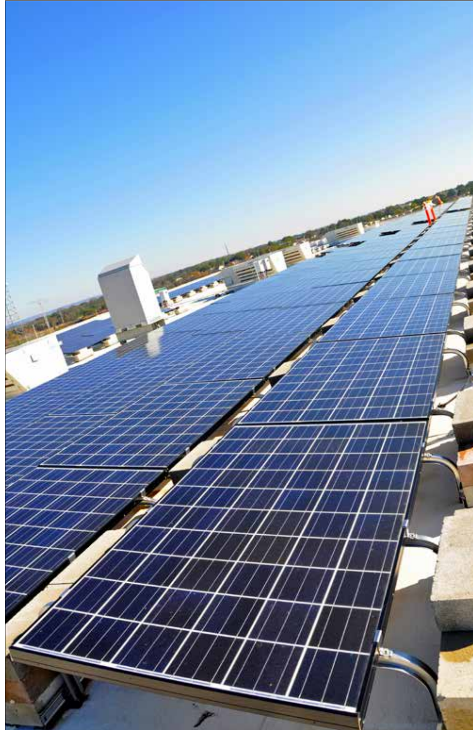
Solar panels at the Alabama National Guard Joint Force Headquarters building in Montgomery, Alabama, provide clean energy and lower utility costs.
