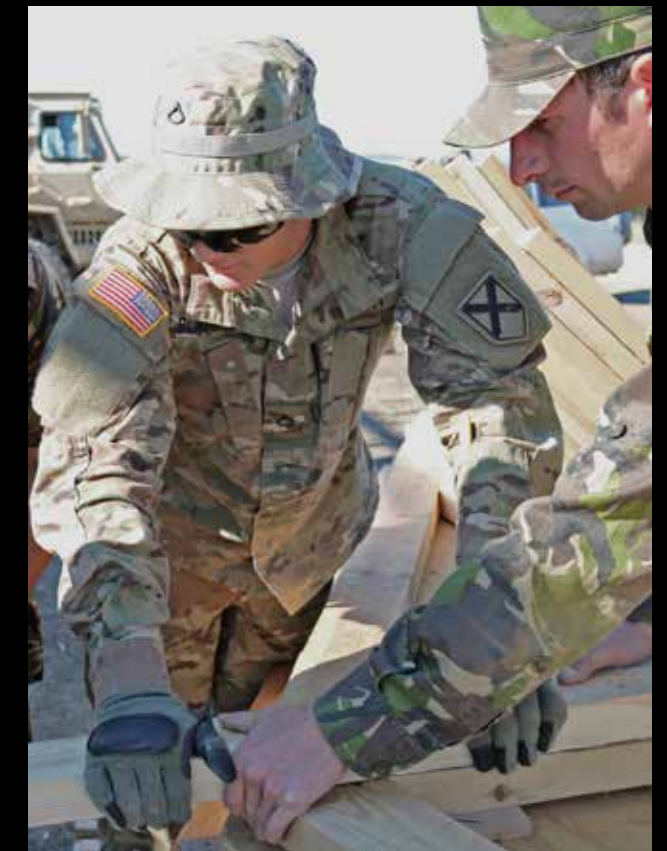
Pfc. Micheal Blackwelder, a carpenter with the 1151st Engineer Company, assists Romanian Soldiers with cutting support beams for an ammunition storage building Aug. 25, 2015, at Cincu Training Center, Romania. American and Romanian forces are worked together in support of Operation Resolute Castle 15. (Photo by Staff Sgt. Fredrick Varney)
