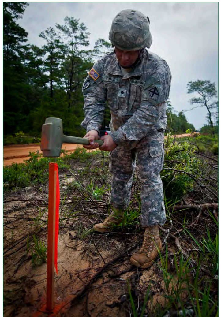
Spc. Craig Davis, of the 1305th Survey and Design Unit, drives a stake into the ground to mark the boundary of the road widening along Range Road 219 July 22 at Eglin Air Force Base, Fla. (Photo by Samuel King, 919th Special Operations Wing, Air Force)
