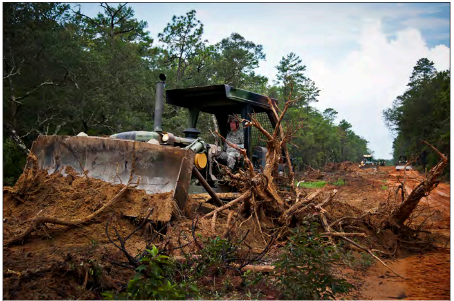
A soldier, from the 877th Engineering Battalion from Alabama National Guard, uses a bulldozer to clear away debris to widen Range Road 219 July 22 at Eglin Air Force Base, Fla. The work saved Eglin approximately $176,000. (Photo by Samuel King, 919th Special Operations Wing, Air Force)
