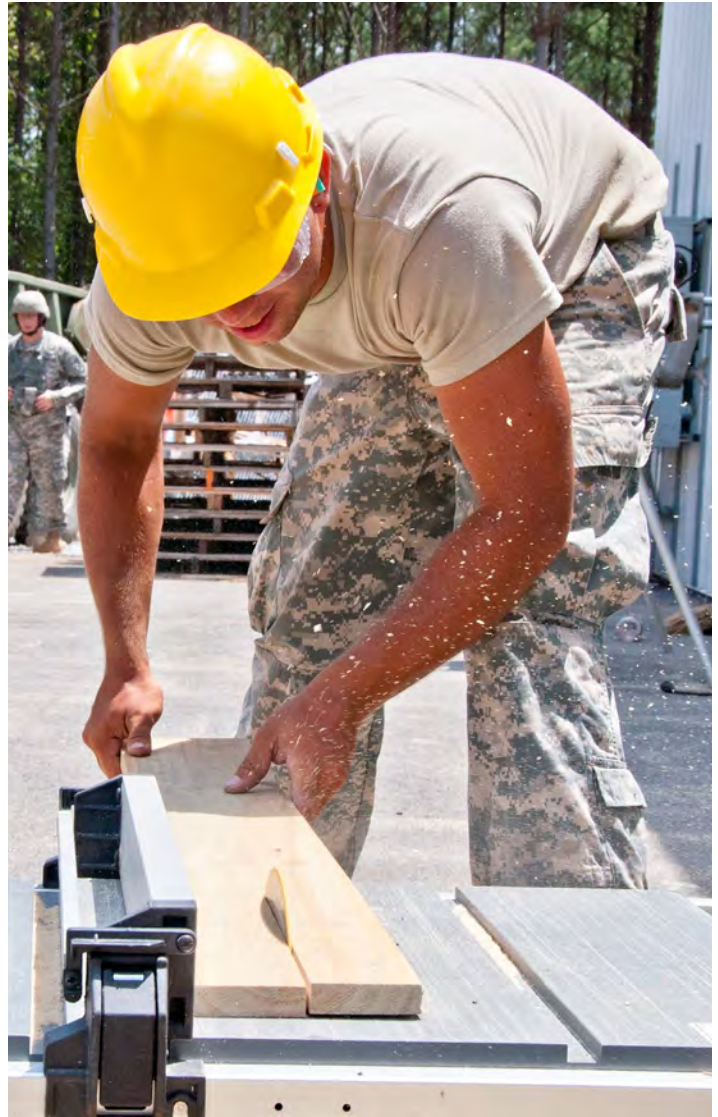
A member of the 1151st Engineer Co. cuts wood to help construct a soffett as part of his annual training exercise. (Photo by Sgt. Brenda Thomas, Public Affairs Office.)
