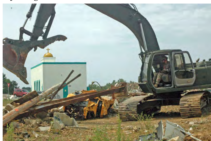
A Soldier helps clean up debris left after a storm. (Photo by Spc. Jonathan Wood, 131st MPAD)
