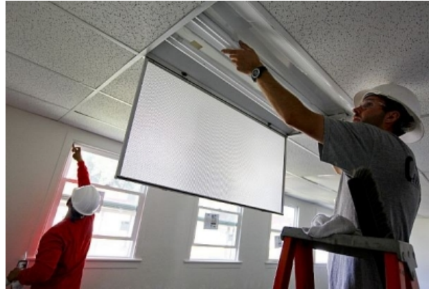
100809-N-8863V-061 NORCO, Calif. (Aug. 9, 2010) Construction workers install new energy-efficient windows and lighting in Bldg. 519 at Naval Surface Warfare Center, Corona Division. Renovations include insulation of exterior walls, water-conservation plumbing fixtures and use of recycled materials. (U.S. Navy photo by Greg Vojtko/Released)
