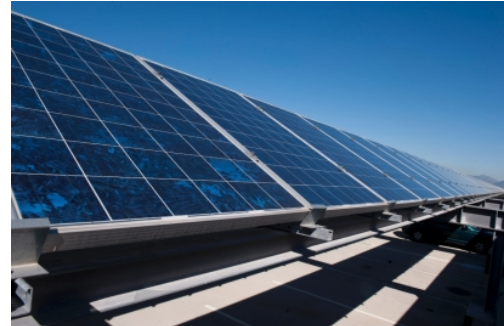
131017-N-ZE250-002 NAPLES, Italy (Oct. 17, 2013) A view of Solar panels installed on top of a parking garage at Naval Support Activity Naples Capodichino. (U.S. Navy photo by Mass Communication Specialist Seaman Weston Jones/Released)
