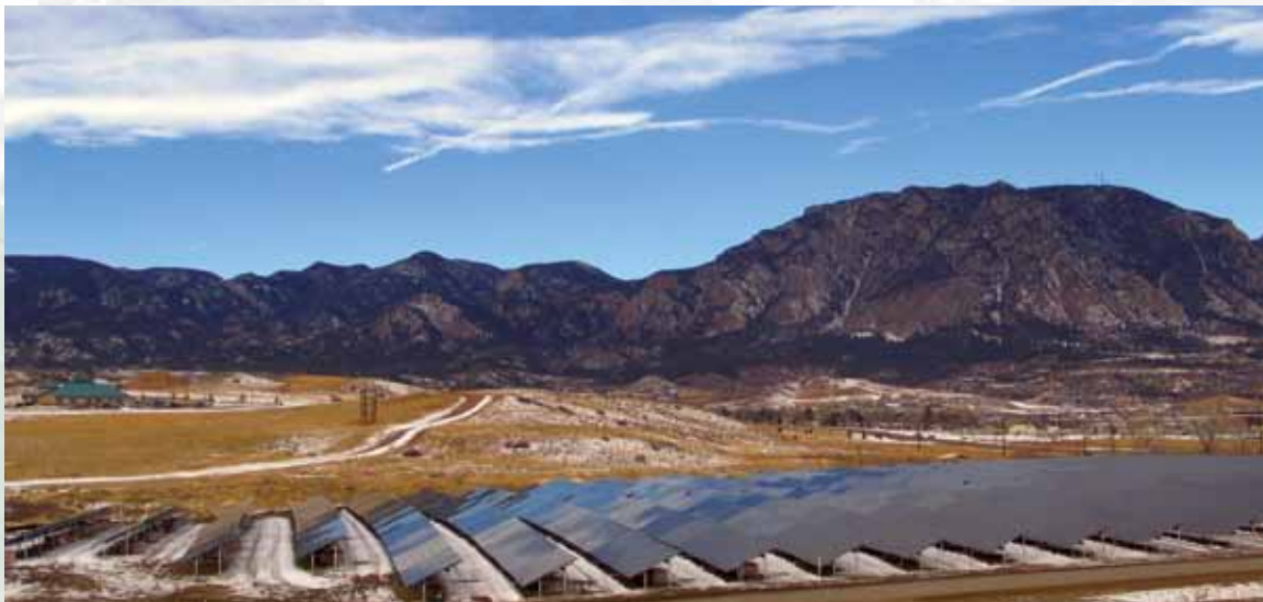
Covering nearly 12 acres, the solar photovoltaic array at Fort Carson is the largest solar array at a U.S. Army facility and one of the largest in Colorado.
