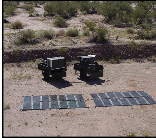
Figure 6 Thin Film Solar Panels with Field Generators
