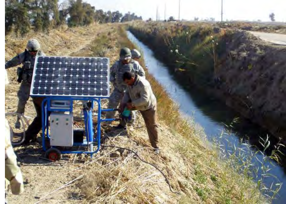
Soldiers from Multi-National Division - Baghdad, 1st Battalion, 63rd Combined Arms Battalion, 2nd Brigade Combat Team, 1st Armored Division, and residents of Chaka 1 work to install a solar powered water filter in Chaka 1, Lutifiyah Nahia on December 16, 2008, to bring clean water to this rural village. Photo taken by US Army, December 16, 2008.
