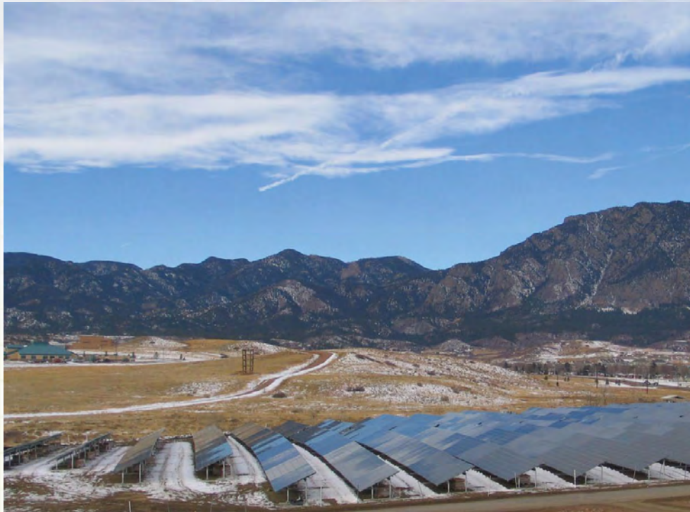
Army's Largest Solar Array Generates More Than Power The Army's largest solar array, a 2-megawatt system at Fort Carson, CO, that should produce enough power for 540 homes.
